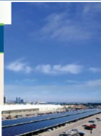
The Naval Base Coronado's solar power system, financed through an ESPC, is one of the largest federal solar power installations in the nation. The solar installation covers an impressive half-mile parking structure and is made up of 3,079 photovoltaic panels.
