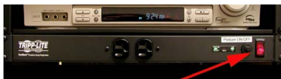
MAIN POWER SWITCH
