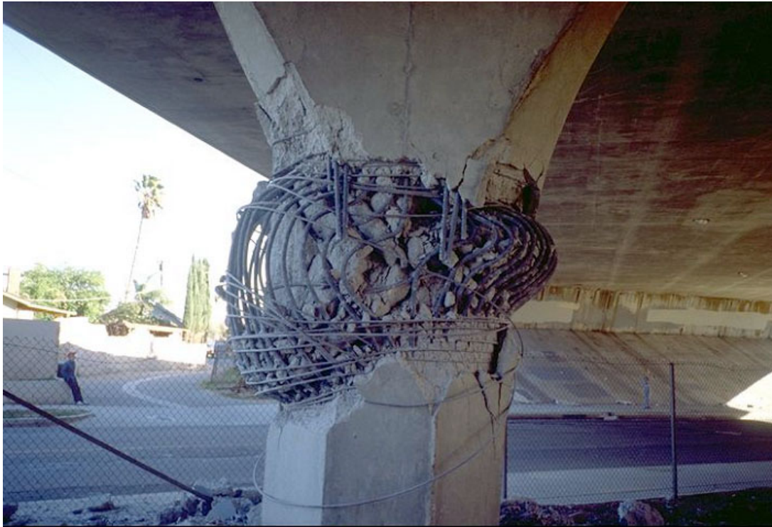
Figure 1.1 Failed bridge column due to the 1994 Northridge, California shallow, crustal earthquake (ACE-MRL, 2013).
