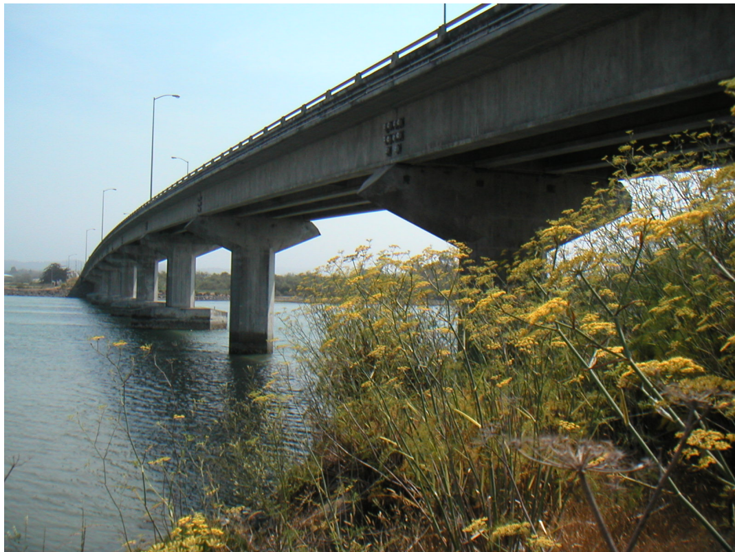
Figure 2.8 View from shoreline of the Humboldt Bay Middle Channel Bridge (courtesy of California Department of Transportation (Caltrans, 2000)).
