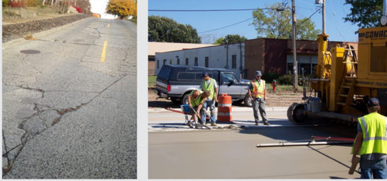
Figure (left) Deteriorated Concrete Pavement; (right) Construction of New Concrete Pavement Containing Recycled Concrete
