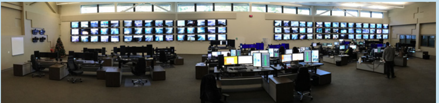
The Northwest Region Transportation Management Center (TMC) at City of Shoreline.
