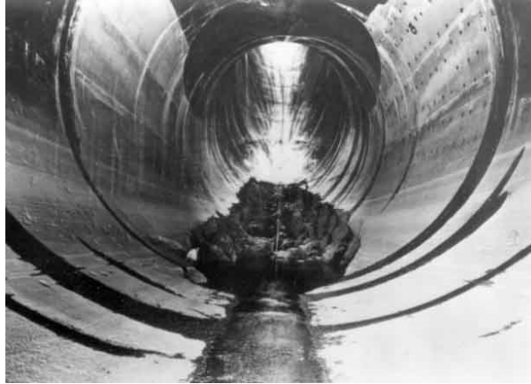
Figure 4.2: Catastrophic failure in the concrete wall of the 15.2 [m] diameter Arizona spillway at the Hoover Dam caused by cavitation.
