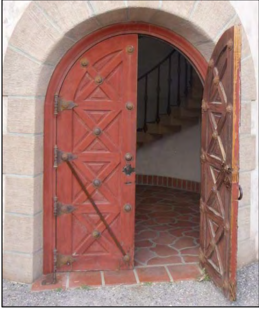
02AE1DO004 before repair
