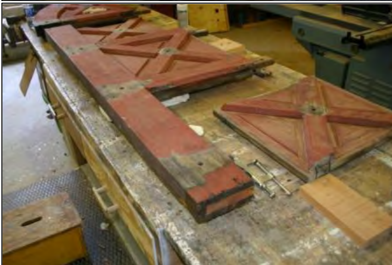
Right-hand (east) stile and bottom rail removed. Stub tenon at lower end of X-munt visible (lower right).
