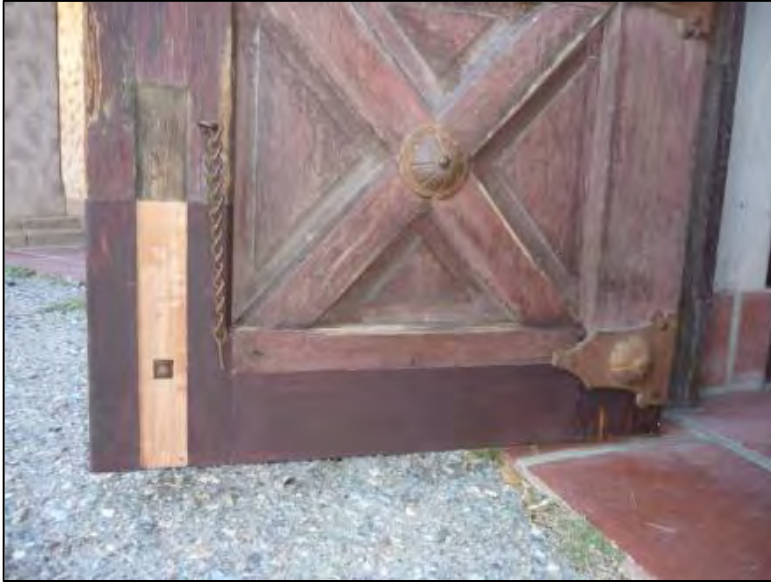
The assembled door showing stile and rail repairs on the door interior at time of reinstallation.
