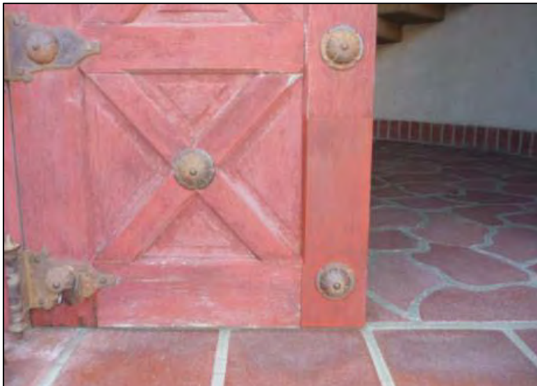
The assembled door showing stile and rail repairs on the door exterior at time of reinstallation.
