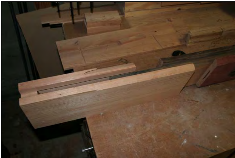
Dutchman extension of east stile prior to assembly. Note the 'biscuit' mortises to strengthen half-lap connections at joint shoulders. The end of the tenon in the historic stile forms the upper mortise shoulder in the repaired assembly.
