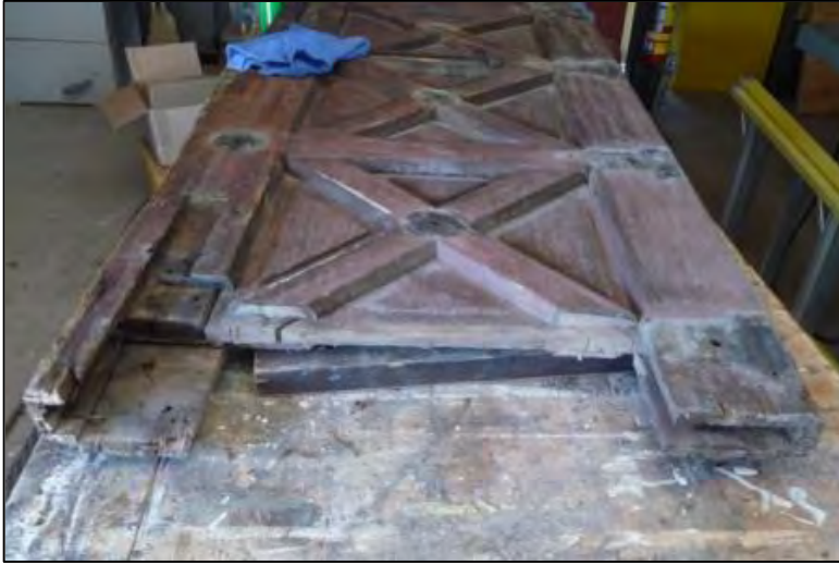
Large loss at east stile-bottom rail connection (bottom left). Bottom rail has been removed.
