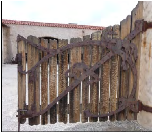
110W1GA002, West face before treatment
