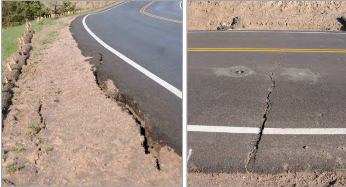
Photo 22. Damage to the Cedar Pass Road in a geological slump area after heavy rain (photo by Brian Kenner, NPS, 2011).
