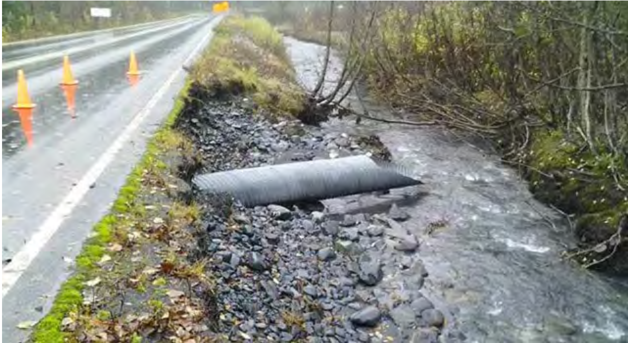
Photo 12. Flood damage and undersized culvert under Exit Glacier Road in KEFJ (Photo courtesy of Western Federal Lands Highway Division, U.S. Dept. of Transportation) (WFLH 2013). The channel along the side of the road in this image is represented by a straight stream channel path displayed in Plate 29.
