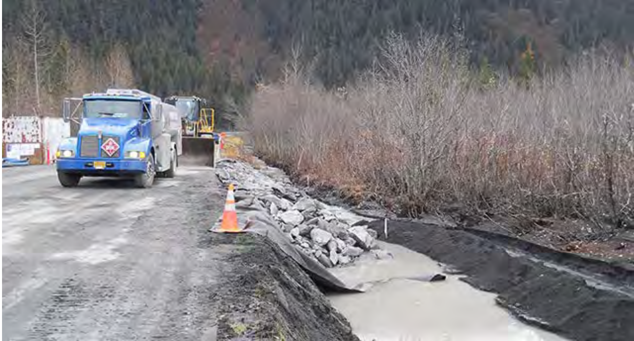
Photo 13. Riprap installation along Exit Glacier Road just upstream from Exit Creek’s confluence with the Resurrection River, October 2012. (Photo courtesy of Western Federal Lands Highway Division, U.S. Dept. of Transportation) (WFLH 2013)
