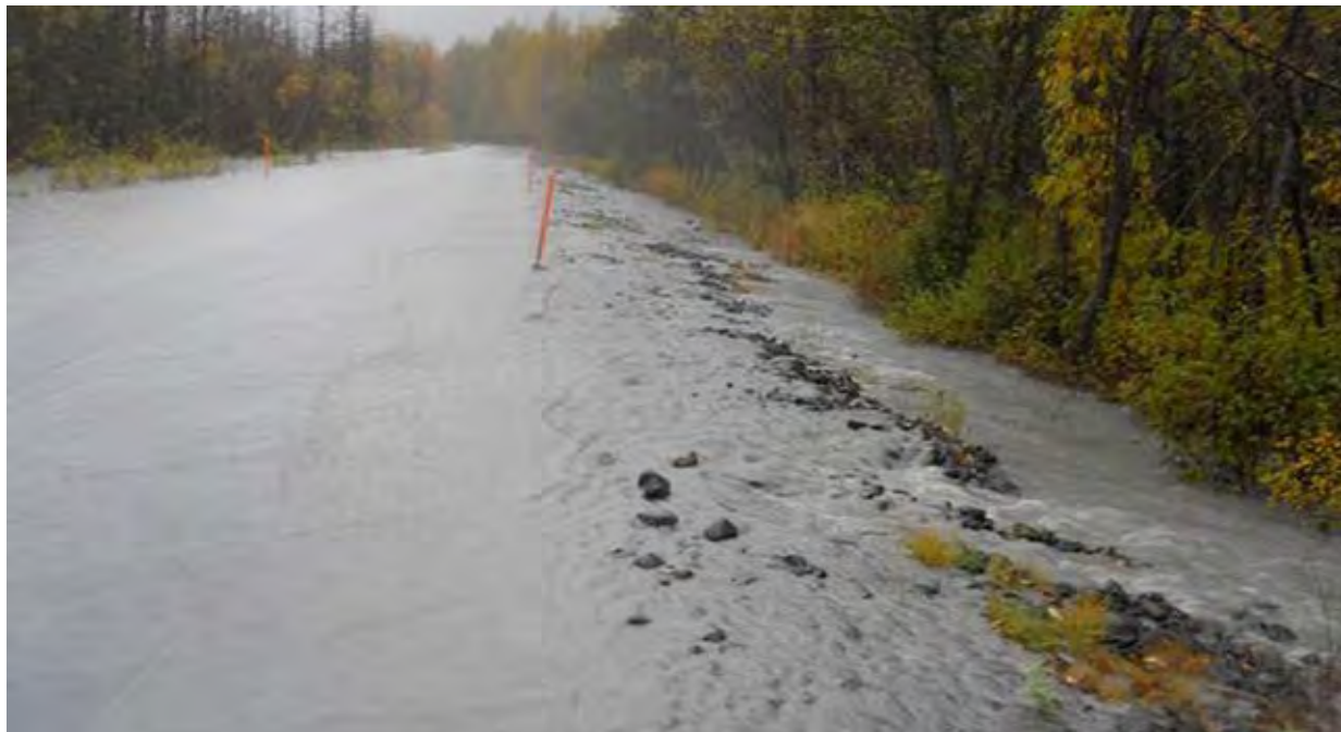
Photo 11. Example of over-road flooding on Exit Creek Road in KEFJ, just west of the Resurrection River Bridge at Exit Creek. (Photo courtesy of Western Federal Lands Highway Division, U.S. Dept. of Transportation) (WFLH 2013).
