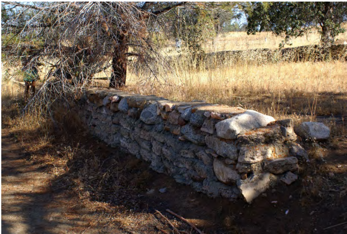
Small-Scale Features: Looking north, an example of a stone retaining wall within the manufactured housing area (PRW, CL Program, 2014).
