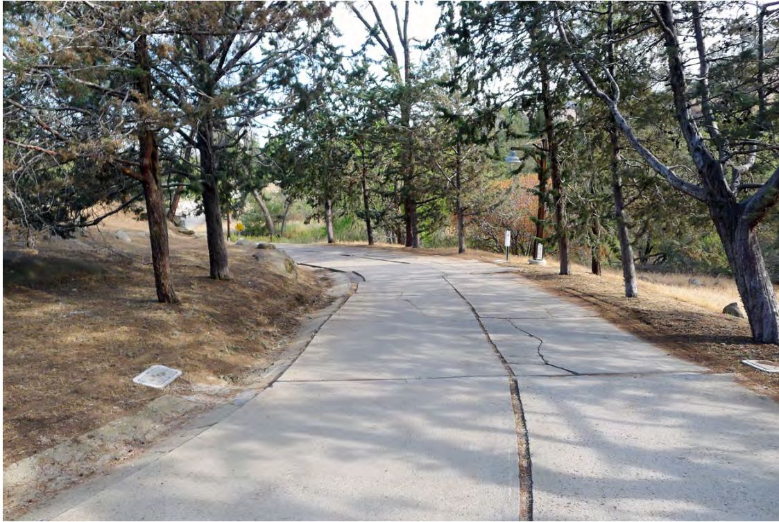
Circulation: The entrance road, looking north to Tehachapi Creek shows the Cypress allée and the road deterioration (PWR, CL Program, 2014).
