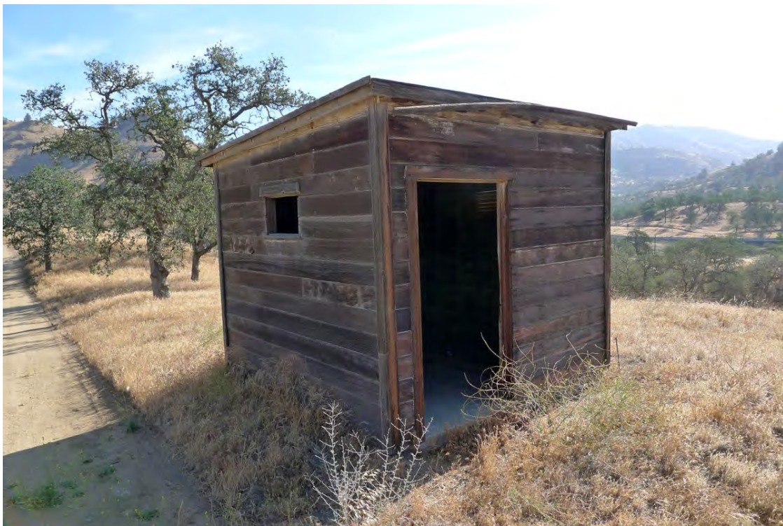
Buildings and Structures: The Hilltop Shack (building 35) located at the top of the hill, and adjacent to the water tower (PWR, CL Program, 2014).
