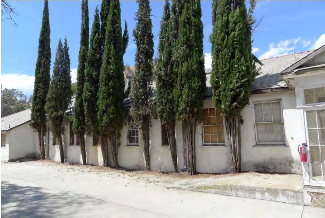
Vegetation: The Dormitory (building 4) building has a row of cypress on the northern side of the building that are encroaching upon the gutter and roof (PWR, CL Program, 2014).
