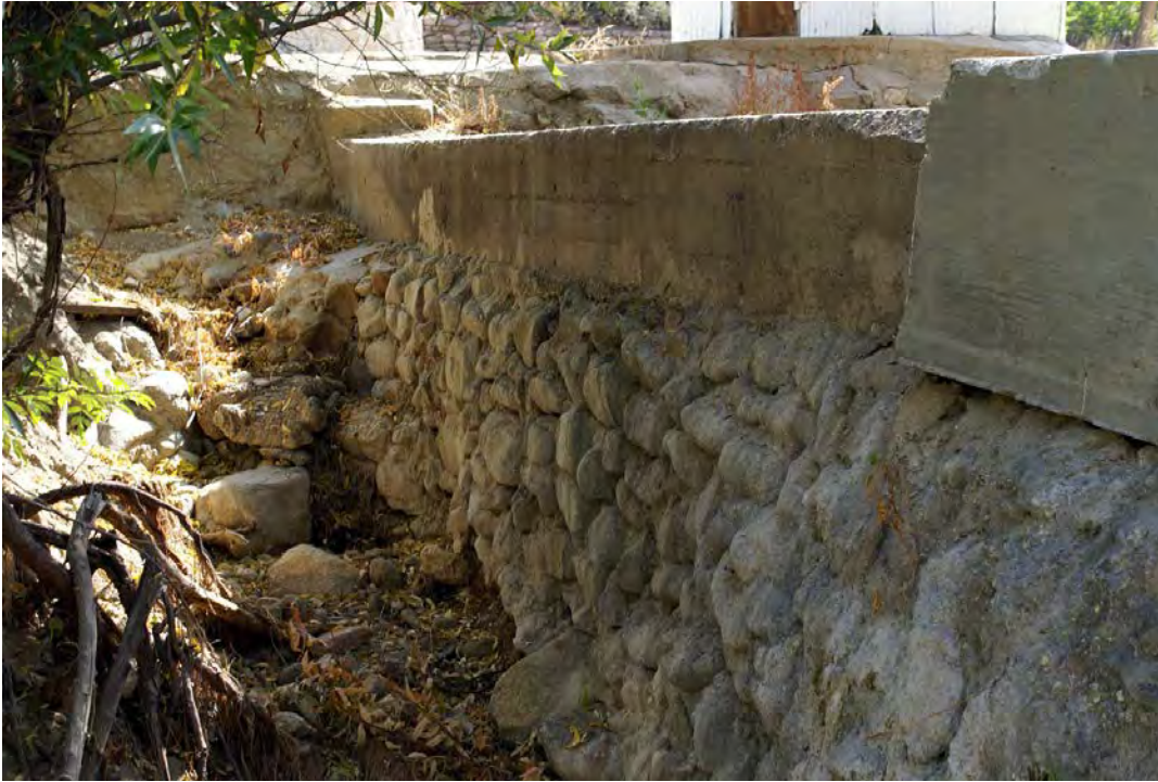
Constructed Water Features: The Tehachapi creek dam, looking east, is located directly adjacent to the South Pump House (building 31) is constructed of concrete and lined with stone on the northern side (PWR, CL Program, 2014).
