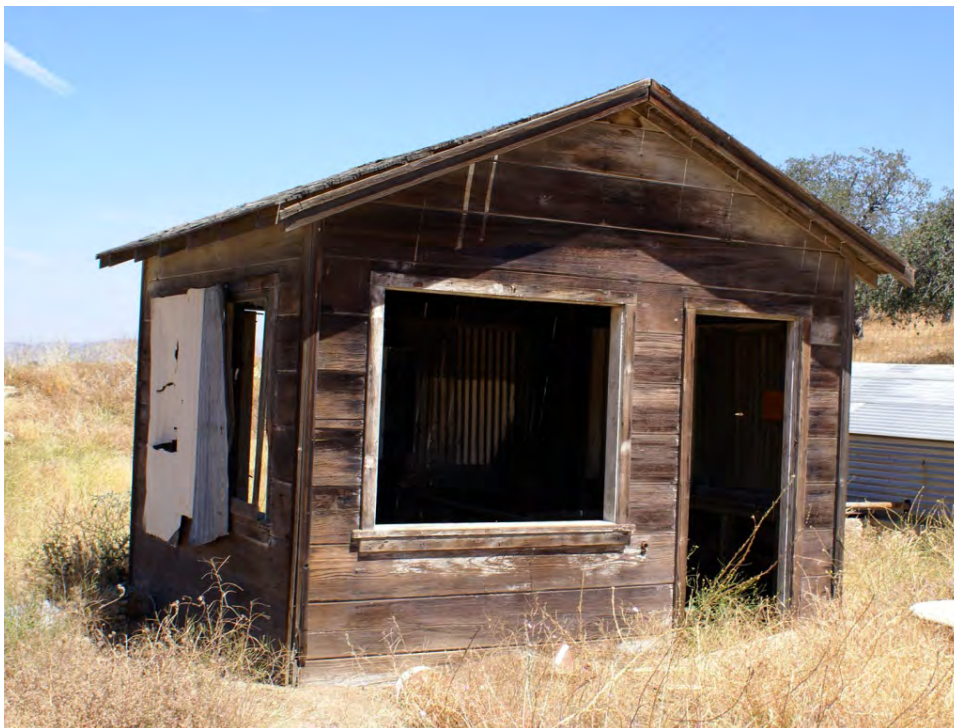
Buildings and Structures: The first settling ponds Pump House 1 (building 33), looking north, at the southern entrance of the pond area (PWR, CL Program, 2014).
