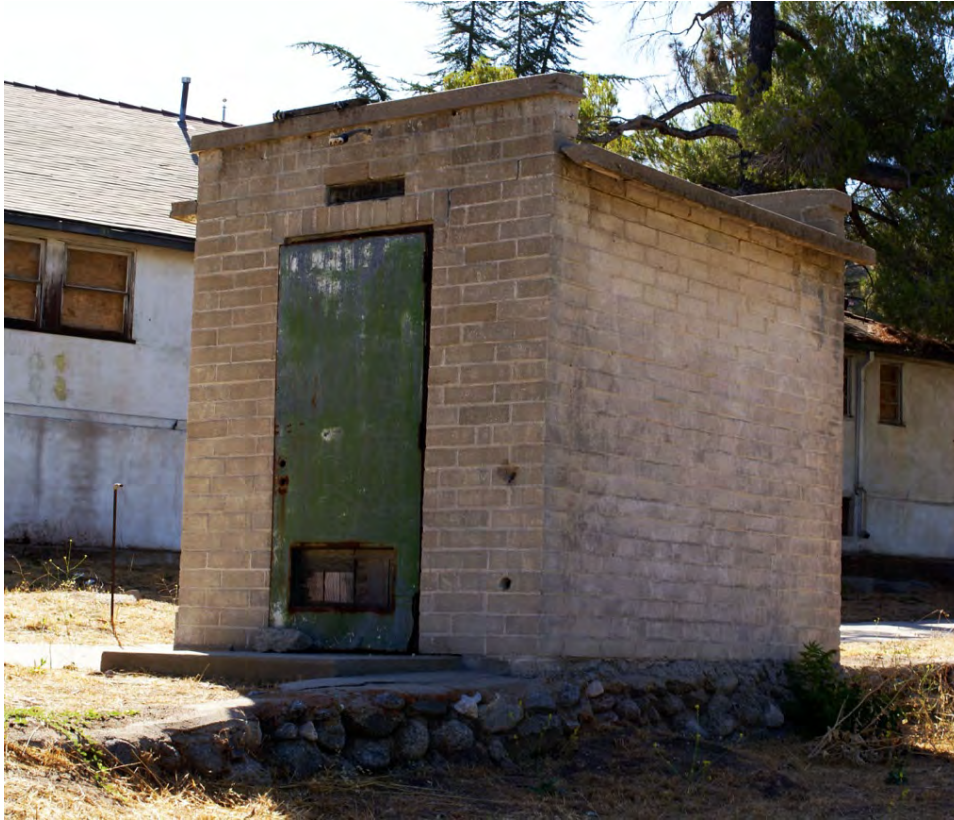
Buildings and Structures: The Boiler Room, located on the southwest side of the Dormitory (building 4), stands on a leveled surface formed by the existing stone retaining wall (PWR, CL Program, 2014).
