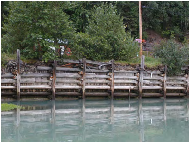
Figure 2-4. Crib wall at Railroad Dock. This crib wall, although it is not itself historic, shows the historical method that was used to construct this wharf out into the harbor, and is an example of a construction method that is similar to the method used to build the original Moore's Wharf before and during the Gold Rush era, as described by Captain Moore. Seen from Small Boat Harbor (July 2004).
