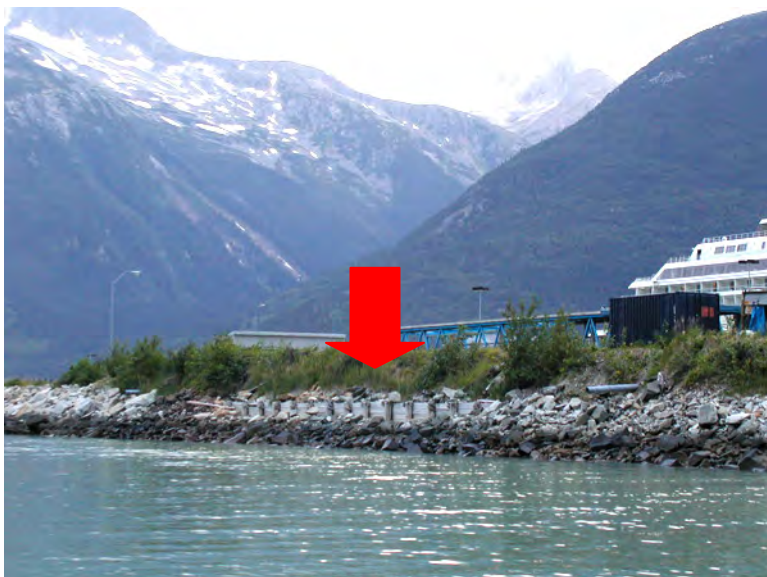
Figure 2-5. Crib wall remnant visible on west side of Small Boat Harbor, partially obscured by rip rap (loose rock fill) (July 2004).
