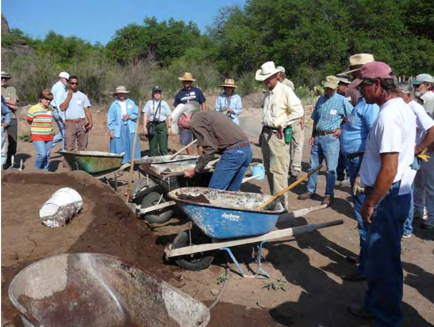
Figure 5. Participants in a workshop, led by Pat Taylor of Cornerstones Community Partnerships, learned about traditional adobe construction and repair.
