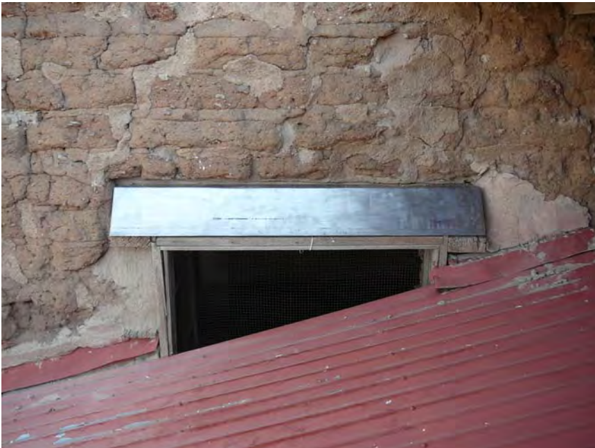
Figure 2. On the exterior of the Kitchen window, a new drip cap was installed.
