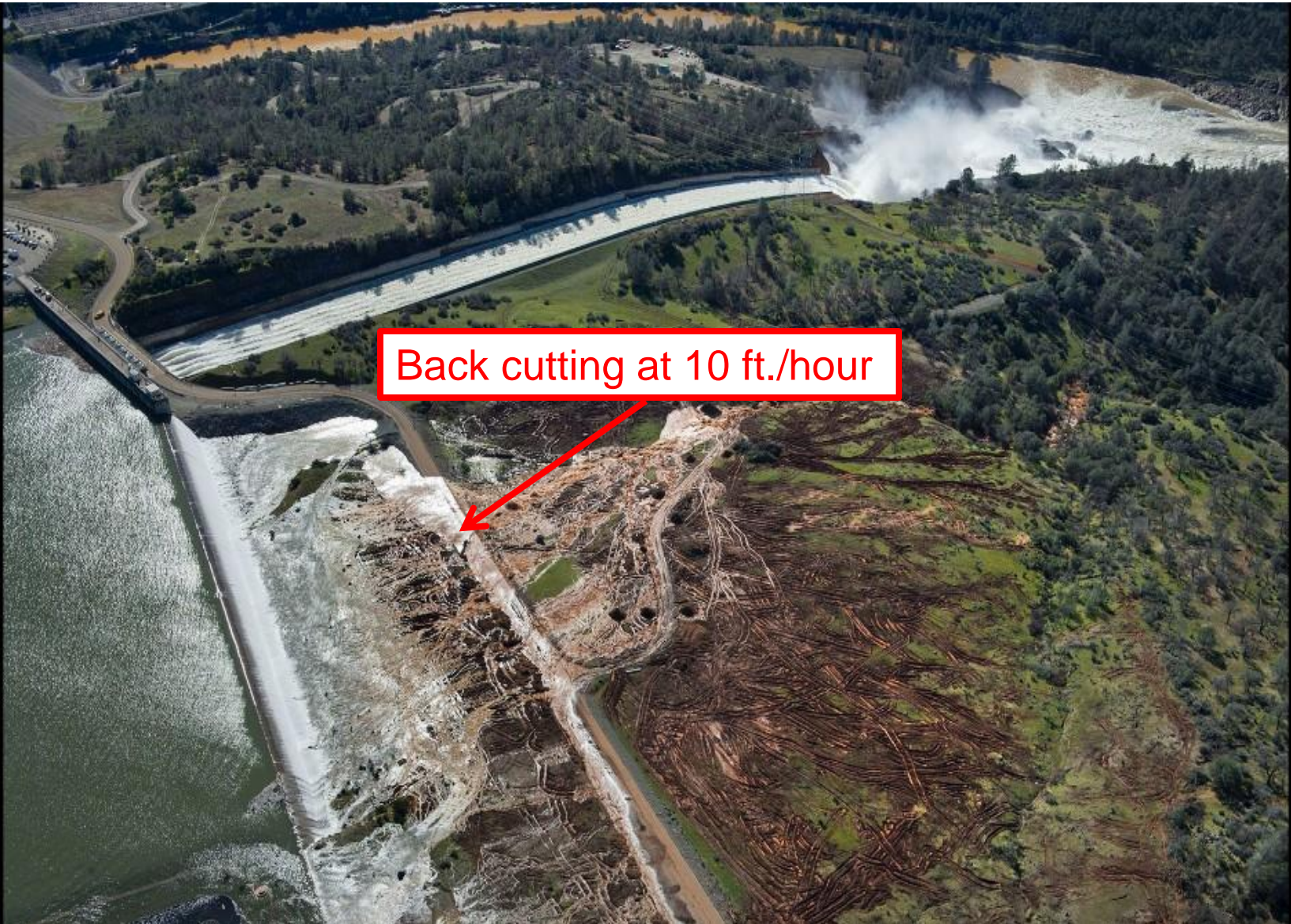
Damage from use of emergency spillway
