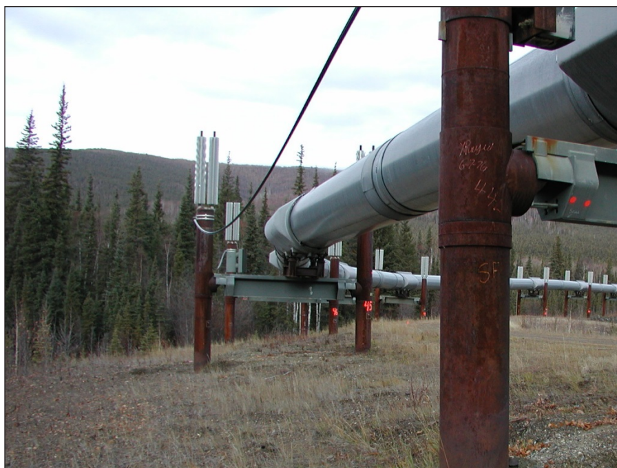
FIGURE 3 The Trans Alaska Pipeline System is elevated above the ground surface over approximately half its length to minimize degradation of underlying permafrost. Thermosiphons are incorporated in the pilings to dissipate ground heat. Photo credit: Doug Goering.
