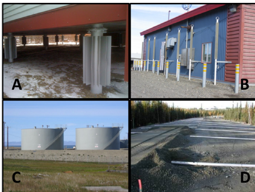
FIGURE 4 Mitigation measures for construction on permafrost at various sites in Alaska. A: Thermopiles supporting raised construction in Bethel. B: Vertical thermosiphons promote passive heat transfer in Kaktovik. C: A gravel pad insulates underlying permafrost from fuel tanks in Kaktovik. D: Horizontal thermosiphons installed in a road embankment in Fairbanks. Photo credits: A, D: Doug Goering; B, C: Yuri Shur.
