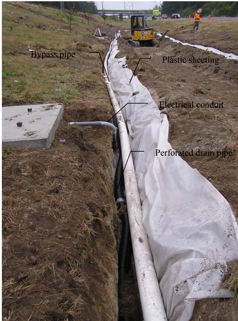
Figure 13. French drain trench with plastic sheet lining, perforated (black) and soild pipe (light), and electrical conduit installed
