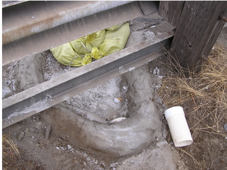
Figure 16. Curb cut and inlet pipe with temporary cap removed and flow blocking sandbags in place
