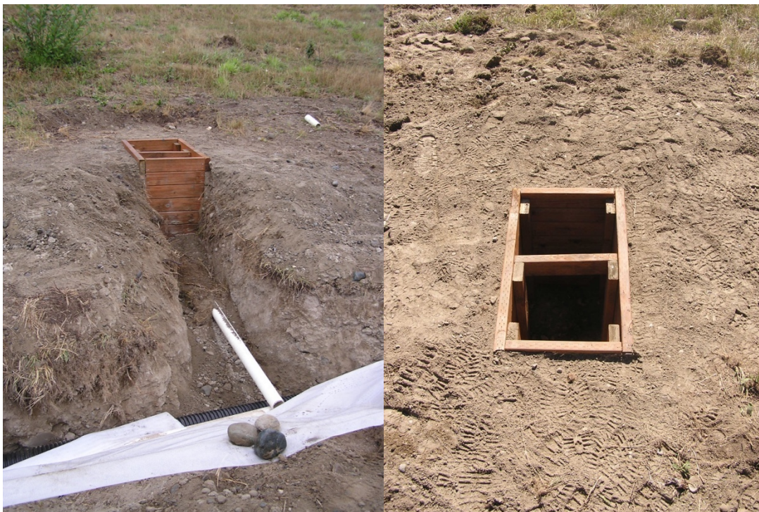
Figure 25. Wood box for TB3 pit rain gauge showing drain to French drain (left) and fully installed
