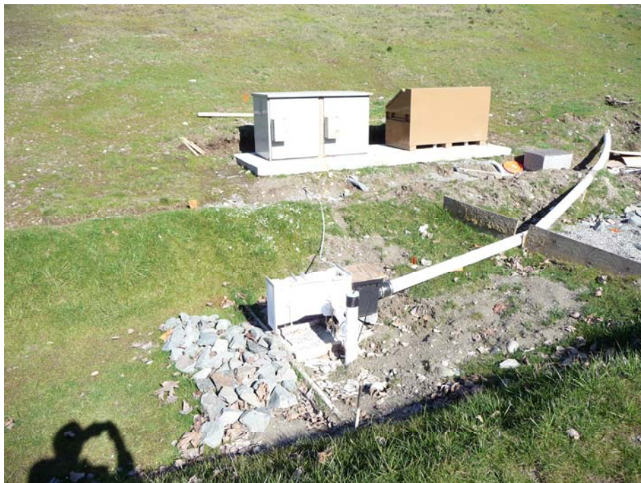
Figure 34. Parshall flume at inlet to bioswale 2
