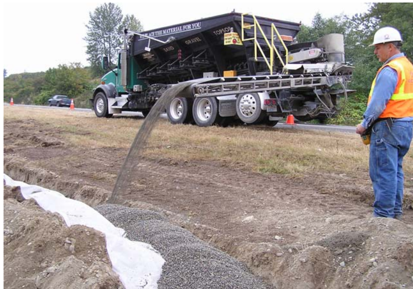
Figure 17. Pea gravel being placed in French drain by an aggregate delivery truck
