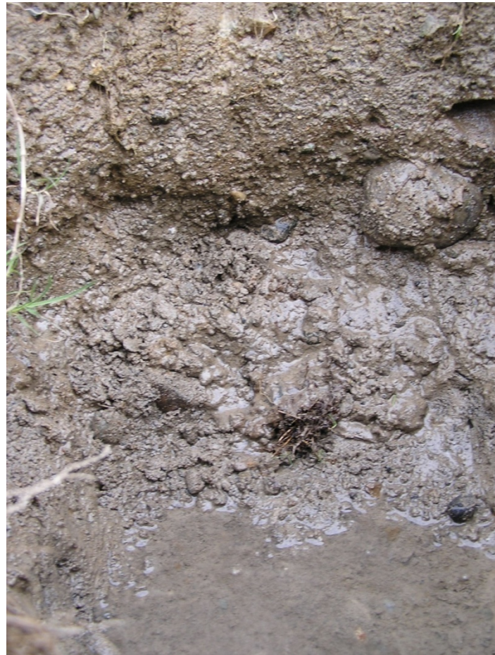
Figure 21. Water seeping from sides of ISCO pit
