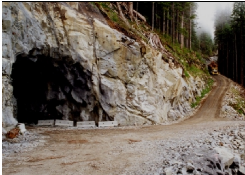
Figure. 3: adit and the railroad-style switchback at the CW 300 road at Phillips Arm. Trucks come down the upper road, back into the adit, and then turn sharply and continue down the lower road at far right. The adit is fully grouted and bolted to minimize rockfall.
