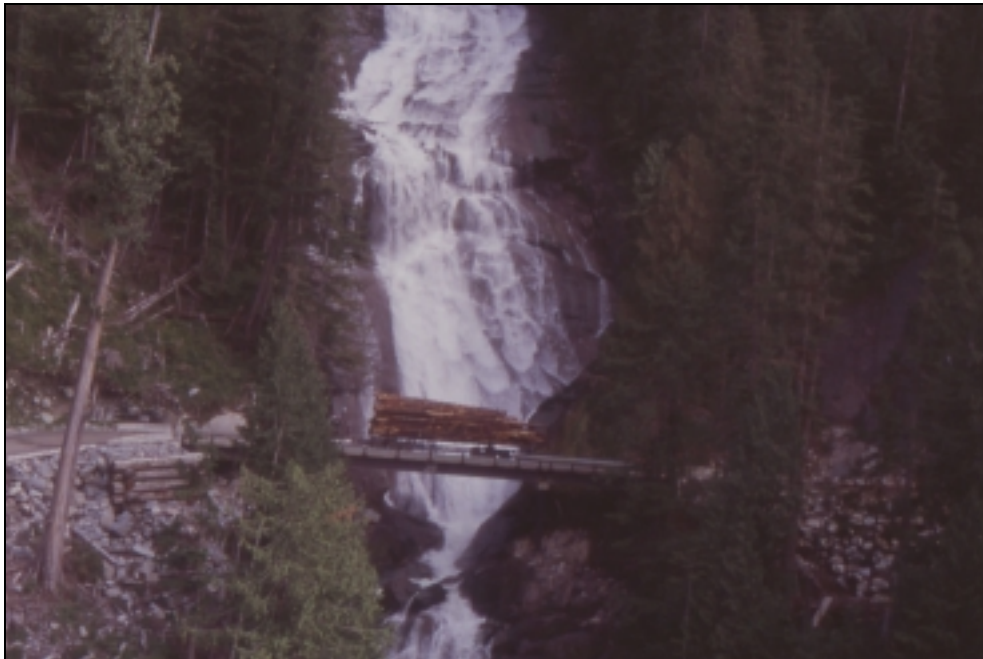
Figure 4: overview of the Shore Creek bridge at the base of the waterfall. In winter, ice avalanches are a major problem at this location and the bridge needed to be designed to avoid being damaged by both high water flows and cascading ice.
