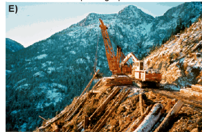
E) View south showing the grapple yarder and loader yarding logs to the stump crib constructed section of road. This is the same section of road shown in (B) and (C).
