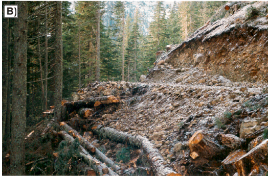
B) View south showing the log crib structure shortly after construction in Fall 1999.
