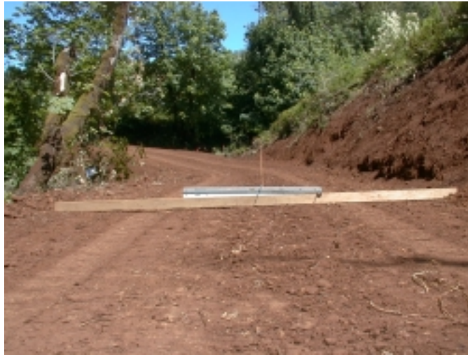
Figure 4. Subgrade of a reconstructed segment being checked for 4 percent outslope with a 3.7-meter (12-foot) board and angled level prior to rocking.
