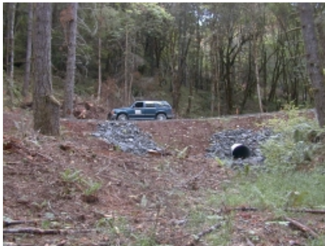
Figure 5. Sag point of the vertical curve offset from the culvert to protect the fill on a relocated section
