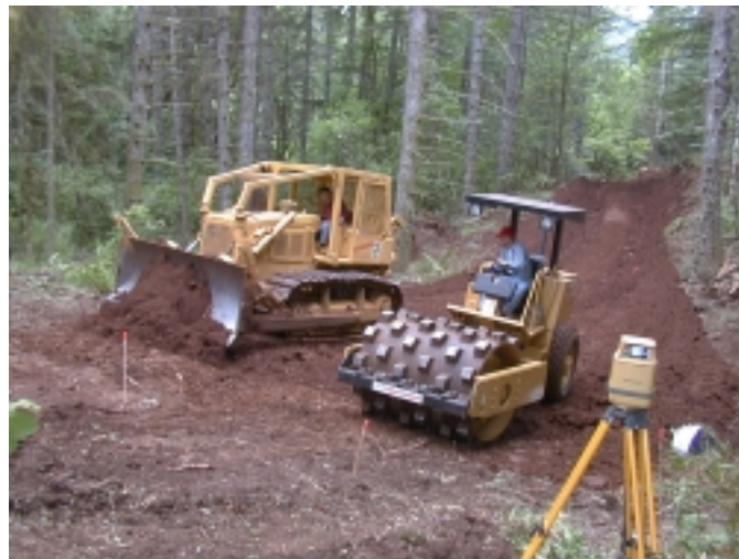
Figure 3. Dozer and sheepsfoot roller work together to bring fill up to grade in compacted layers for sub-grade stability on a segment of relocation.
