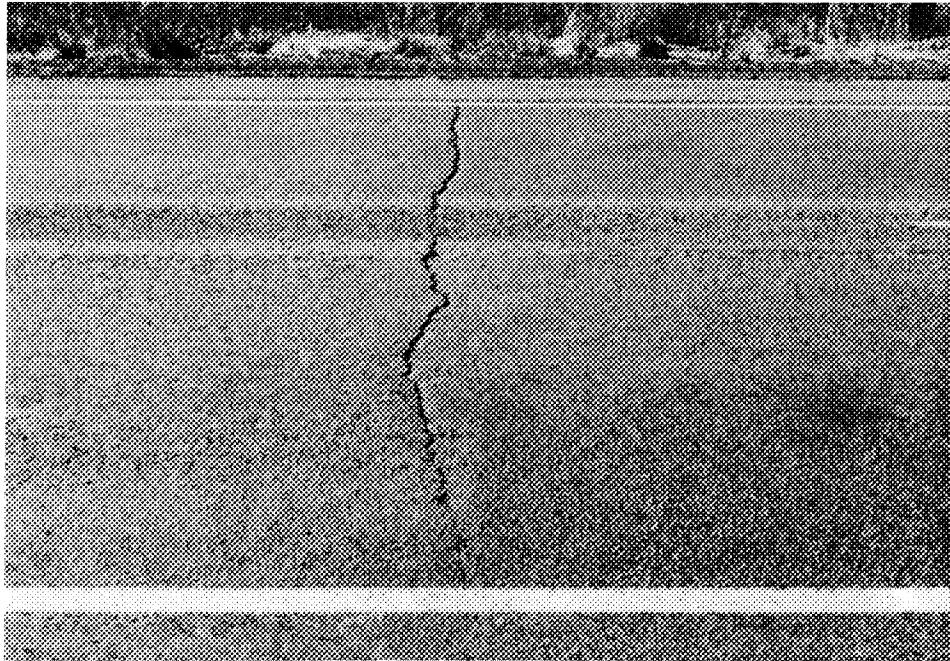
Figure 12. Pre-construction Transverse Crack in Sections B and E
