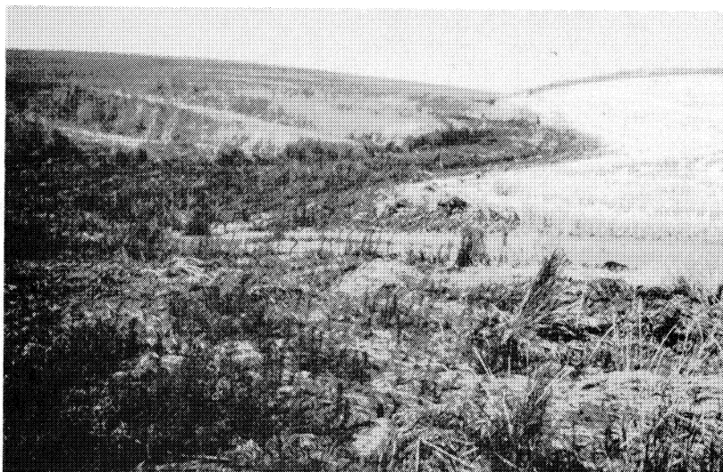
Figure 28. The drainage basin above the piping is relatively large. The lack of an adequate drainage system explains the extensive damage.
