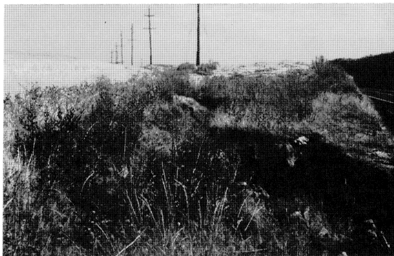
Figure 22. Gully erosion in a side ditch due to insufficient channel protection.
