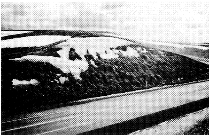
Figure 37. North facing slope opposite the cut in Figure 36 exhibits severe gulley erosion.
