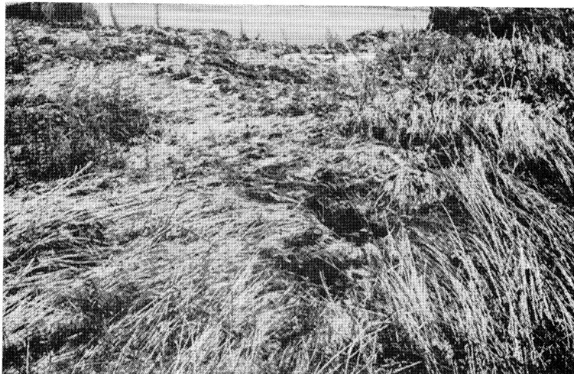
Figure 27. Dark areas below center are piping inlets located approximately 10 feet behind the cut.
