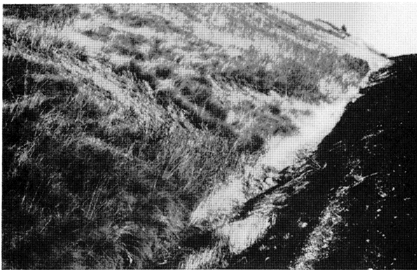
Figure 32. Shallow failures with arcuate scarps are fairly common in silty loess near the eastern extremity of the study area.
