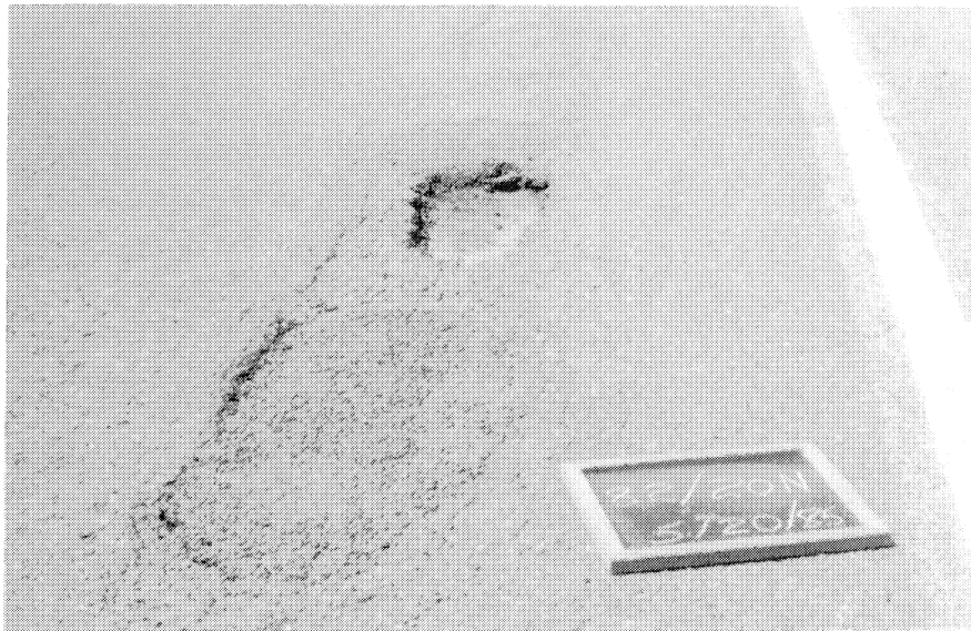
Figure 4. Stripped AC Caused by Defects in the Bottom of the Overlay
