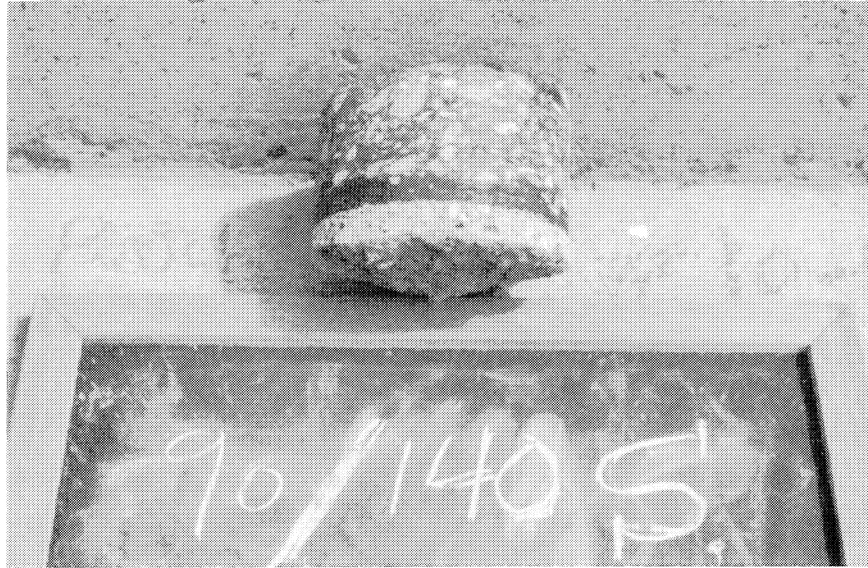
Figure 7. Concrete Delamination (Patch) Under Sound AC Overlay and Membrane.
