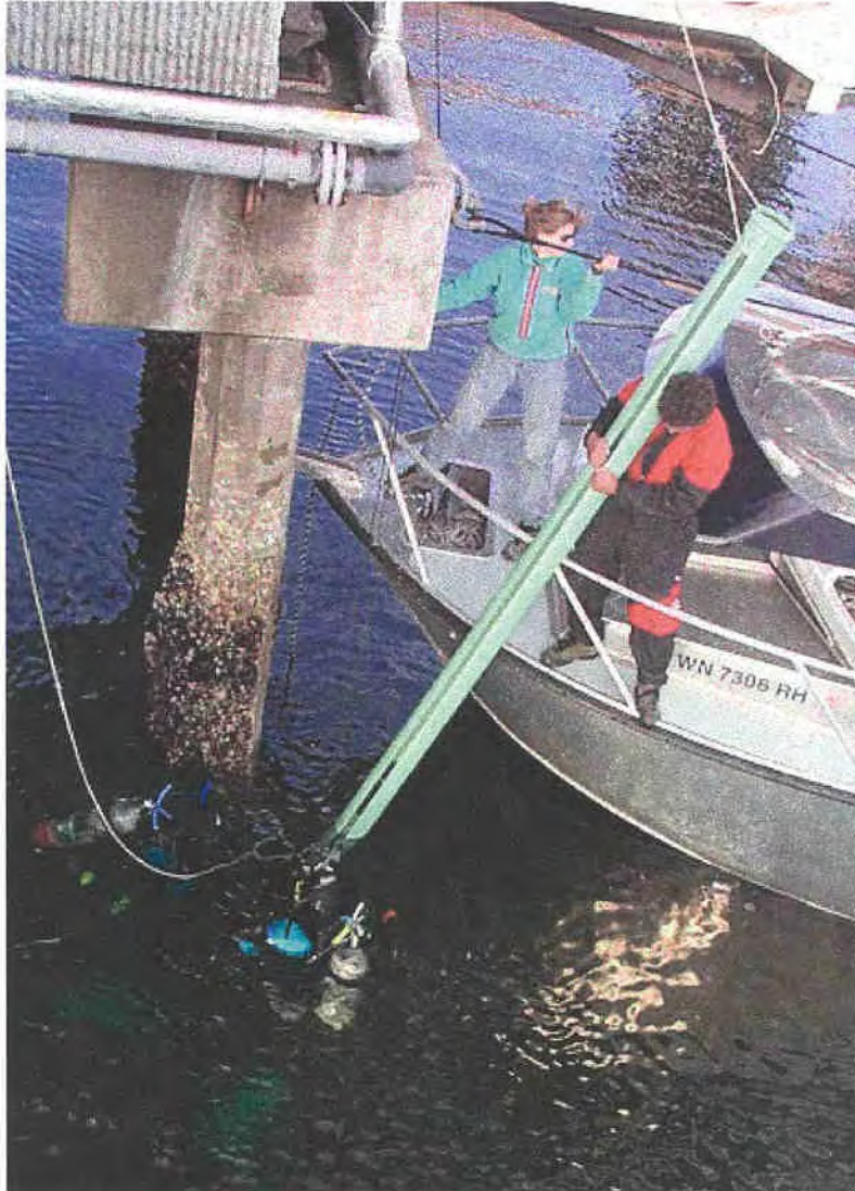
Figure 7. Installation of a slotted polyvinyl chloride (pvc) pipe, which contains two single-beam transducers attached to a sealed pvc float, at the Port Townsend ferry terminal in June 1999
