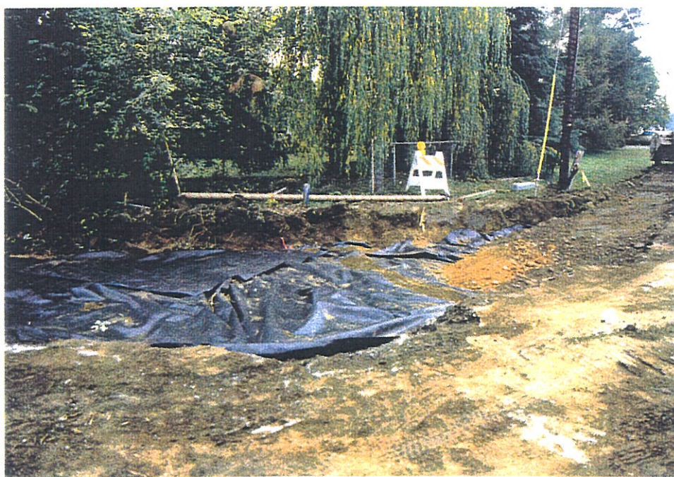
Figure 5.42 - Typical installation procedure for the radius widening areas. Note the backfill placement technique on the far right side (Courtesy of WSDOT).
