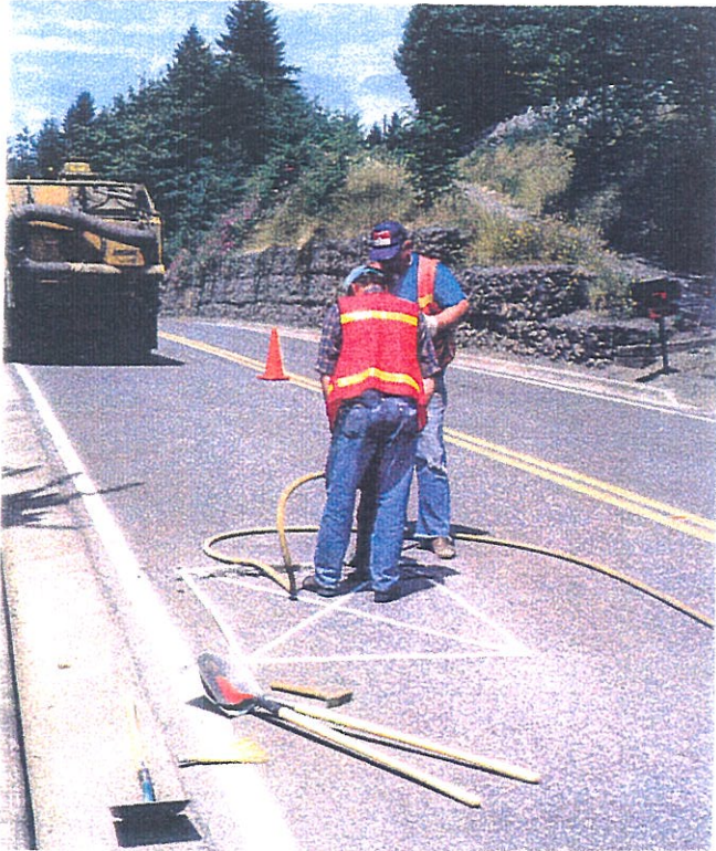
Figure 5.24 - Testpit location for the Pacific Way site, with the ACP being removed.
