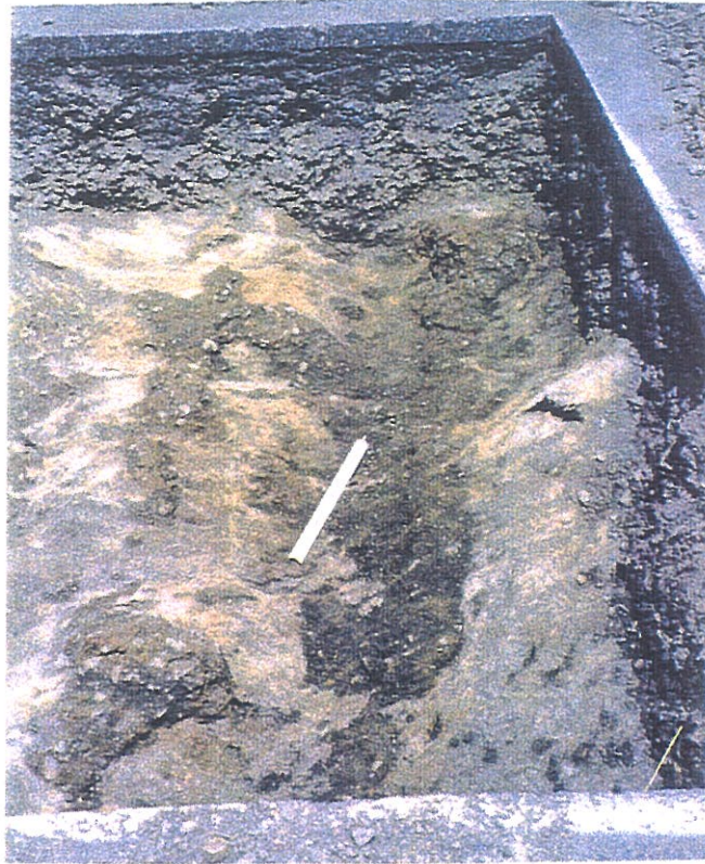
Figure 5.12 - Exposed geotextile and clay protrusions, testpit 1.
