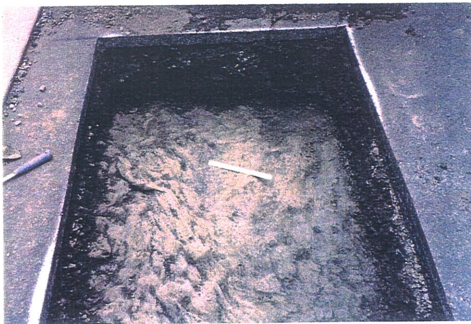
Figure 5.92 - Exposed geotextile. Looking west.
