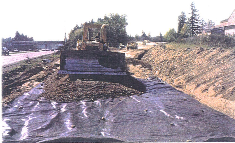
Figure 5.72 - Dozer spreading the initial lift over the geotextile separator (Courtesy of WSDOT).
