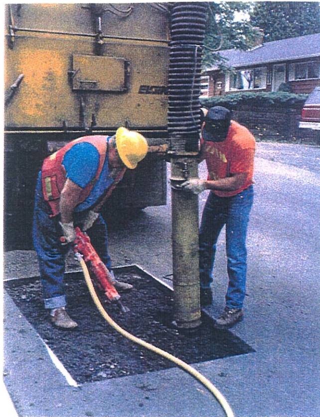
Figure 5.90 - Base being loosened with a jackhammer and being removed with the Vac-all.
