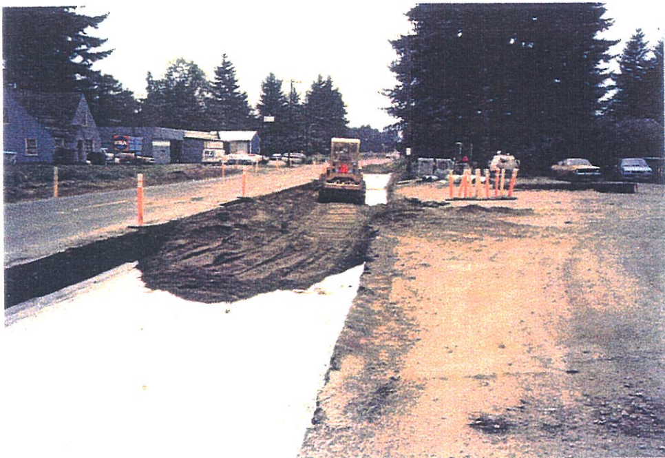
Figure 5.79 - Dozer spreading the initial lift of backfill over the geotextile (Courtesy of WSDOT).
