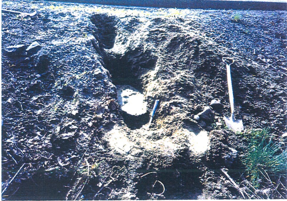
Figure 4.3 - Exposed geotextile separator at Tremont Interchange, SR-16.
