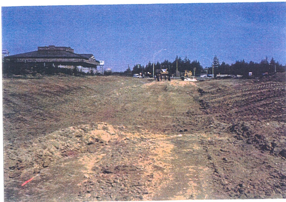
Figure 5.71 - Photograph showing the overexcavated subgrade conditions (Courtesy of WSDOT).
