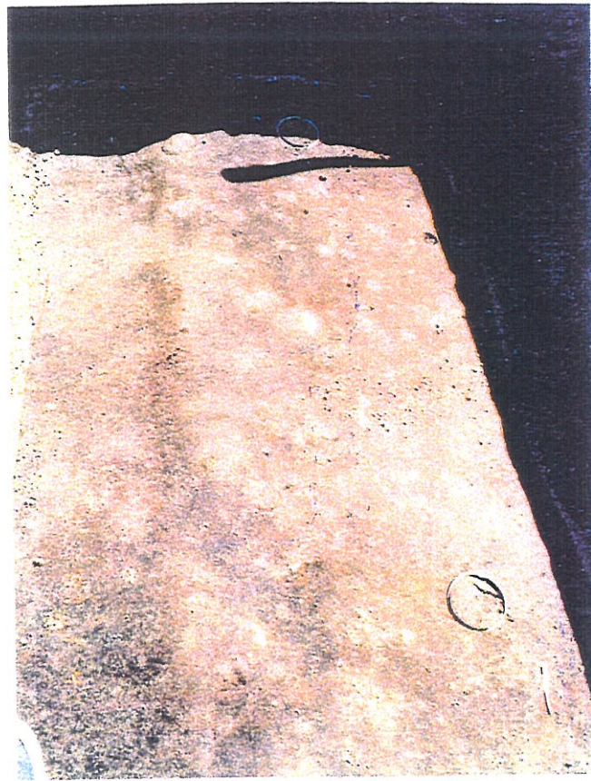
Figure 5.85 - Subgrade surface with the rut shown on the left side.
