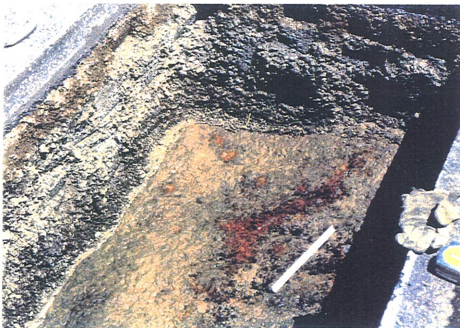
Figure 5.29 - Subgrade surface with iron stained patterns.
