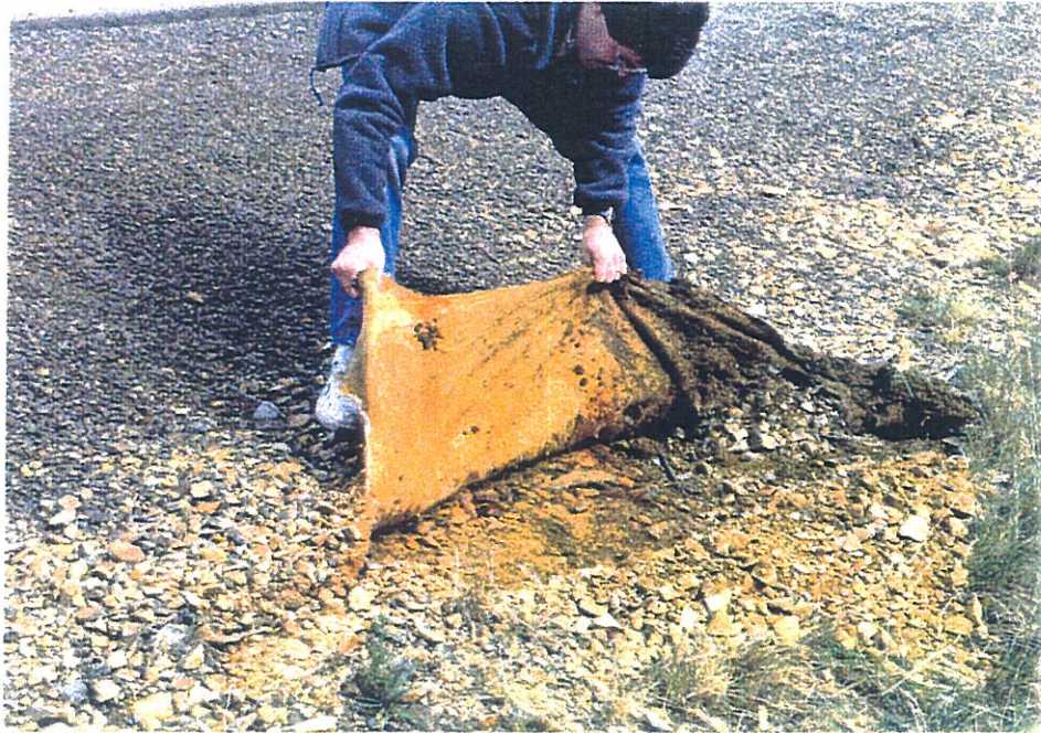
Figure 4.4 - Exposed subgrade under fabric on Parpalla Road.
