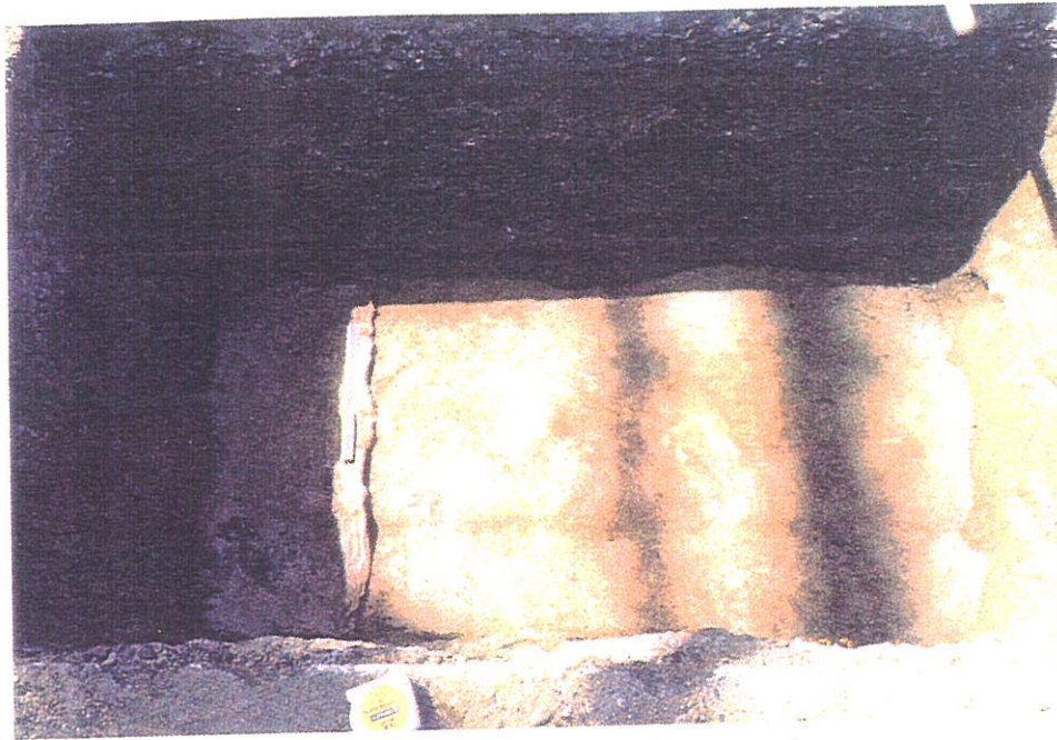
Figure 5.82 - Top surface of the exposed geotextile, showing the overlap on the east side.
