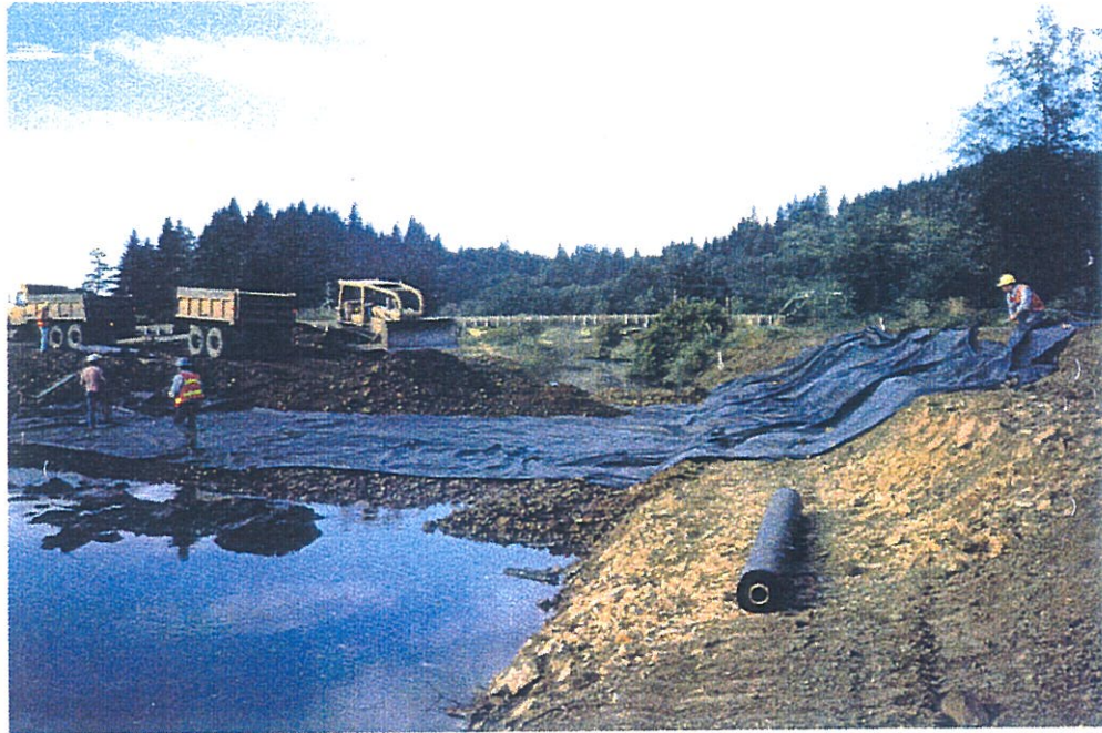
Figure 4.5 - Geotextile being installed in the middle of the embankment during the construction of the Deep River Bridges project.
