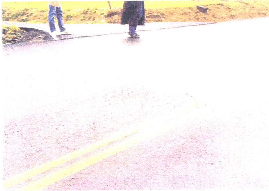
Figure 5.1 - Distressed pavement on Columbia Heights Road.
