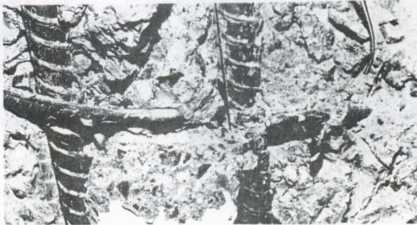
Figure 8 Photographs of Column 3 showing (a) crack patterns at \mu = \pm 2 and (b) rupture of the spiral reinforcement.
