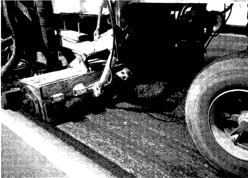
Picture 5. Milling heads of "Unit A". Removes the top inch of heated material. Milling heads remove the outside 5 feet from each side of the travel lane.
