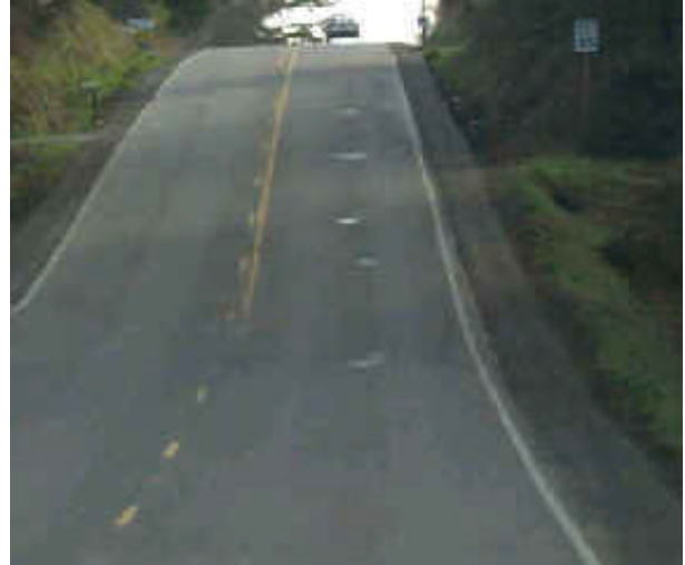
Figure 14. Photo of Low Density Spots.
