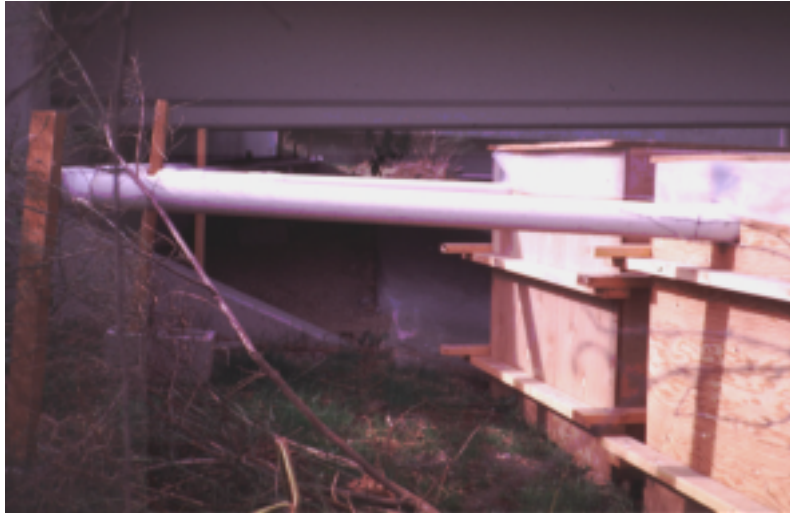
Figure 3.7 Storm water conveyance lines and collection tanks
