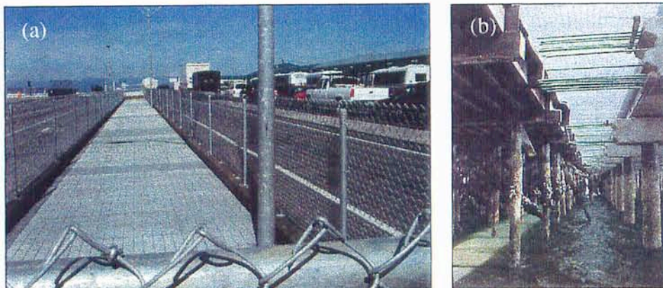
Figure 8. Deck grating from above (a) and below (b) (note the sun/shade pattern on the water surface).
