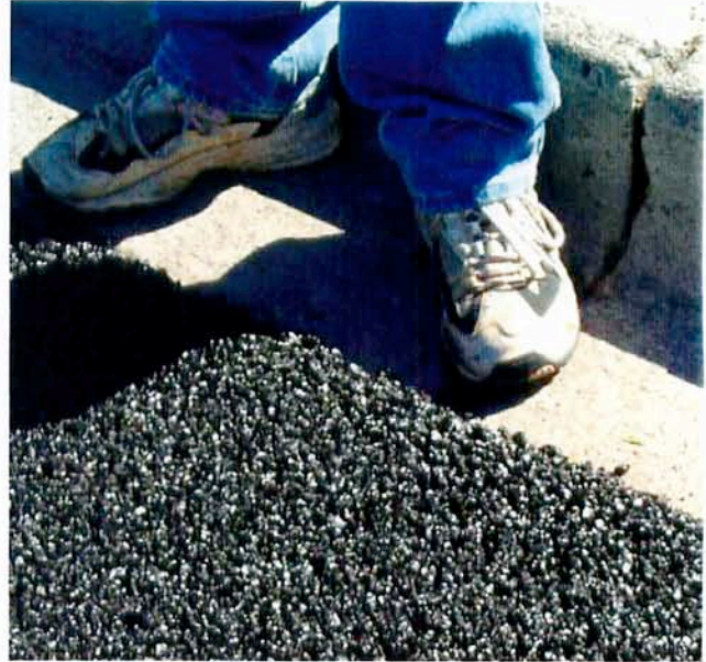
Photo 12. NovaChip® asphalt placed adjacent to curb and gutter. Rotomilling adjacent to the curbing was not done. Previous surfacings and the NovaChip® left a trough in the gutter.
