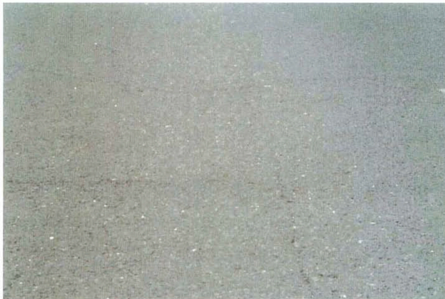
Photo 28. Block Cracking reflecting through the NovaChip ® overlay.
