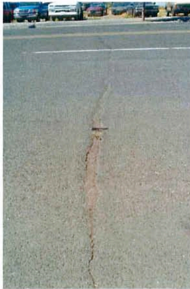
Photo 5. Medium to high severity transverse crack seen on SR 17. Cracks of this width should be crack sealed prior to overlay.
