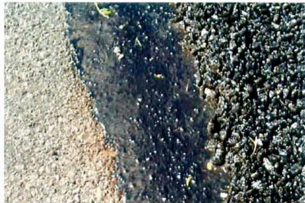
Photo 18. Novabond® Membrane placed outside the hot mix asphalt indicates its heavy thickness.
