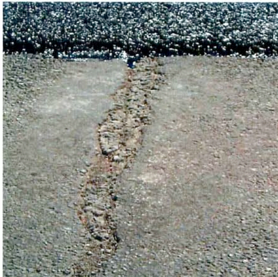
Photo 10. NovaChip® asphalt placed over existing cracks. These transverse cracks should have been sealed prior to the NovaChip®.
