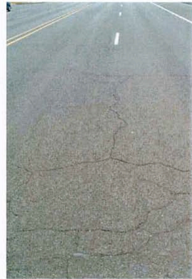
Photo 6. Cracks less than 1/4 inch observed in Soap Lake. Crack sealing or repair is not necessary.
