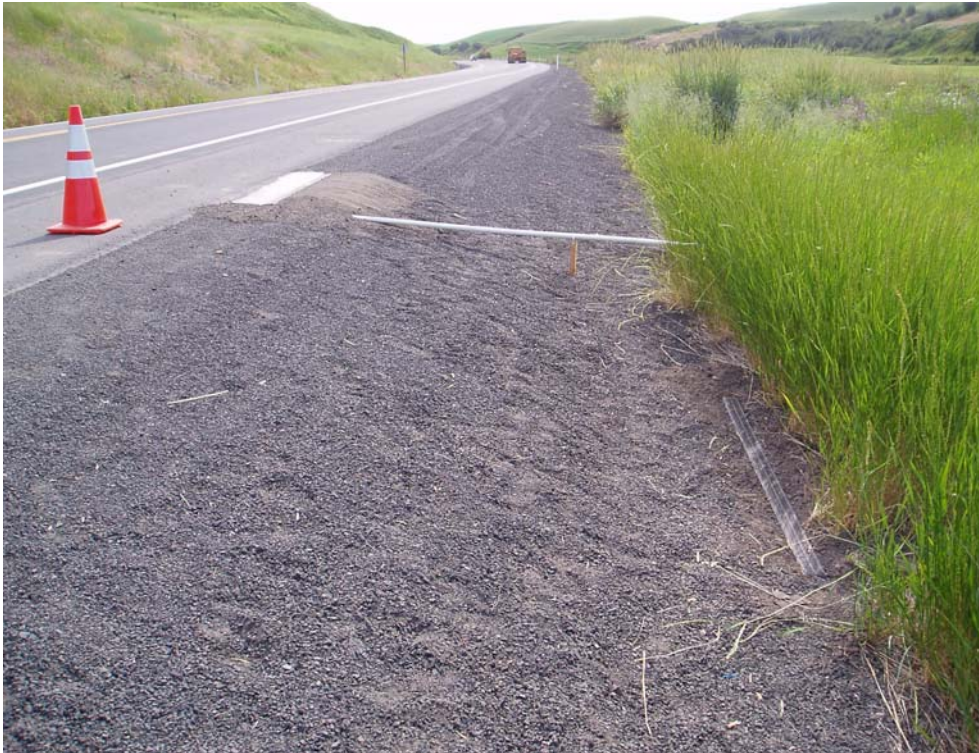
Figure 4. SR-270 Remote Monitoring Site (Pullman)
