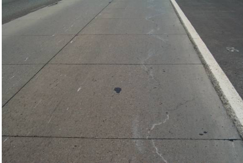
Figure 13. Intersecting corner cracking in the 3 inch ultra-thin whitetopping section. August 2004.
