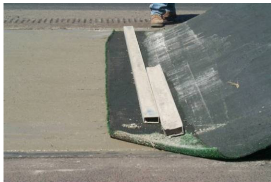
Image E. Close-up of weights use to keep the carpet in contact with the wet concrete.
