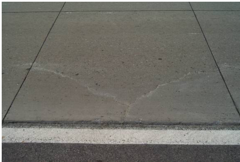
Figure 14. Intersecting corner cracking in the 3 inch ultra-thin whitetopping section. August 2004.
