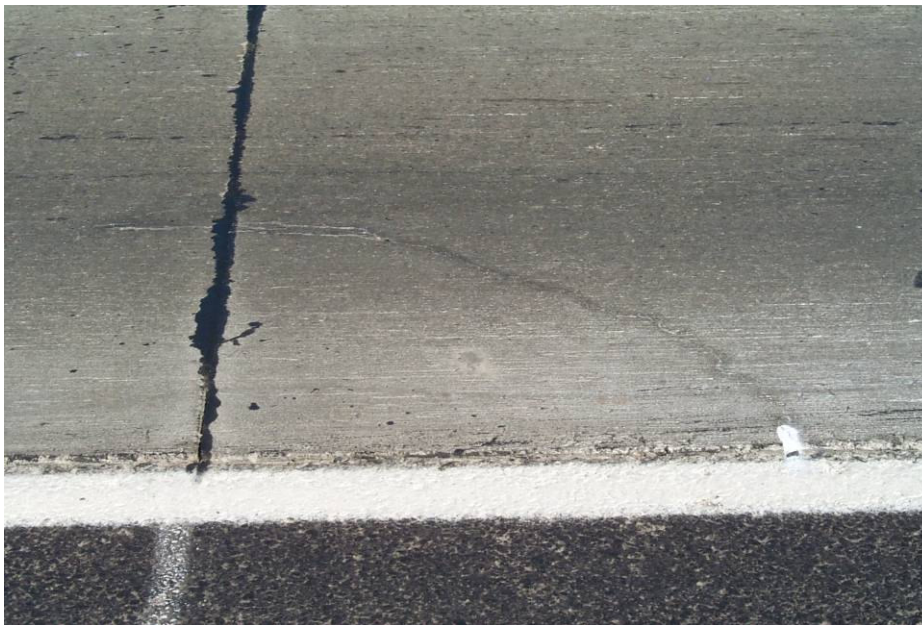
Image 5. Typical corner crack within the 3-inch ultra thin whitetopping test section.
