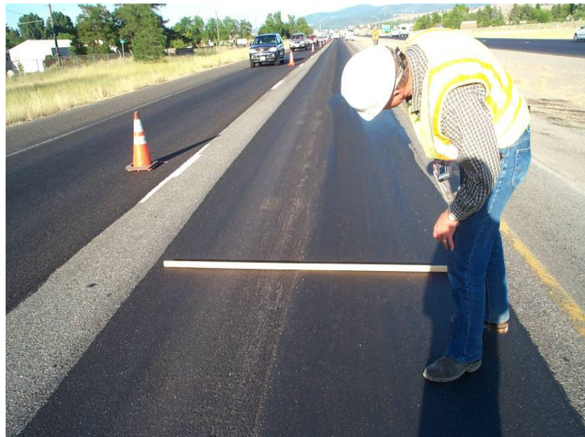
Figure 8. Micro-surfacing placed as a rut fill prior to macro-surfacing within the two westbound lanes of I-90 (MP 293.15 to MP 293.55).
