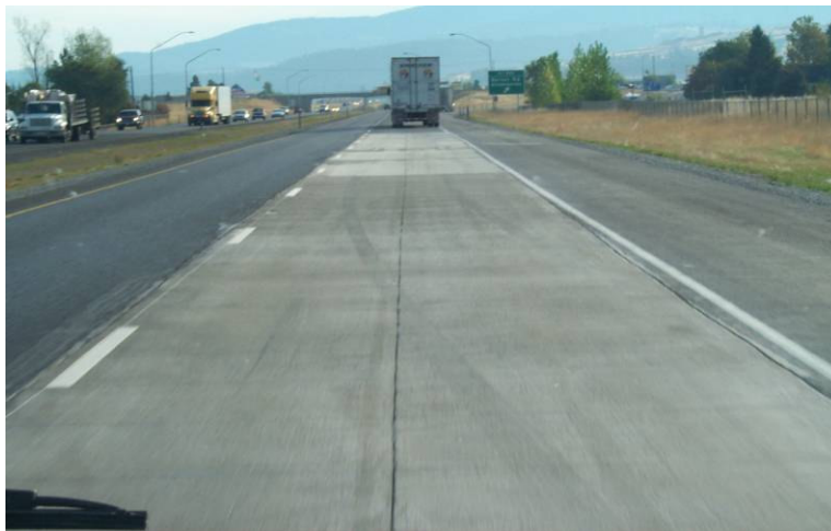
Image 1. Ultra Thin and Thin Whitetopping Test Section placed in the outside lane of eastbound I-90 (MP 293.15 to MP 293.55).
