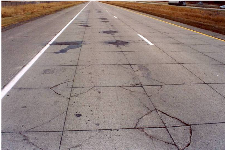
Figure 21. Corner cracking in MnROAD Test Cell 94, 3 inch whitetopping with a 4 ft by 4 ft joint spacing. Photo courtesy of Mn/DOT.
