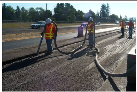
Image B. Cleaning of the existing pavement surface. Note remnants of the Superpave overlay in the wheelpaths.
