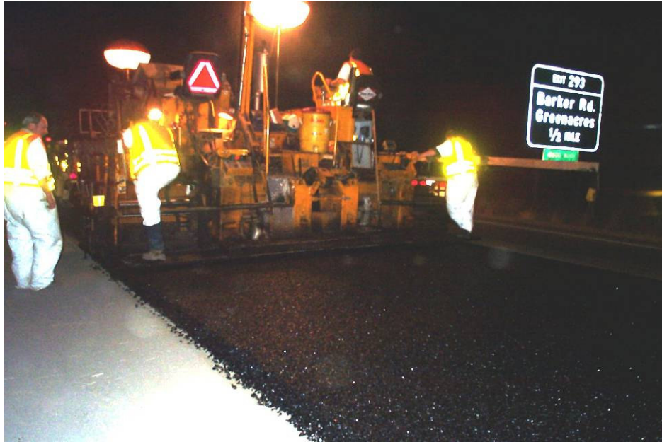
Image 2. Placement of Modified D asphalt in the inside eastbound lane of I-90 (MP 293.15 to MP 293.55).
