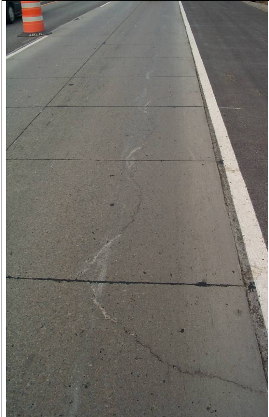
Figure 15. Longitudinal view of intersecting cracking in the 3 inch ultra-thin section. August 2004.
