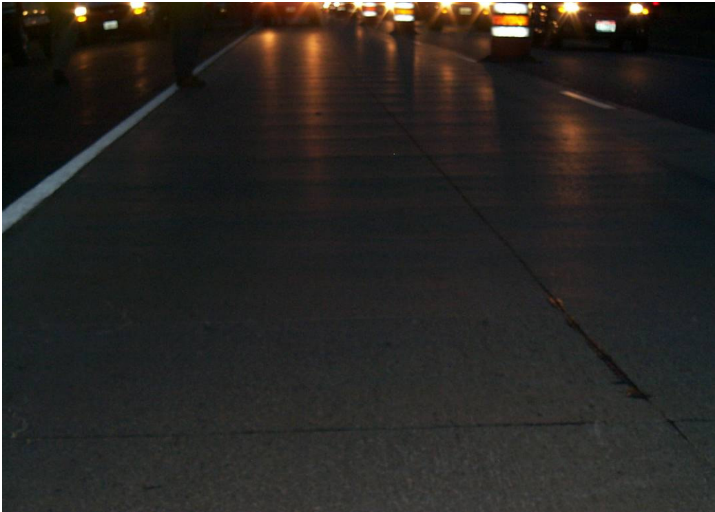
Figure 17. Night time photo of 3 inch ultra-thin whitetopping section showing curling of the panels.
