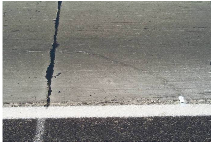
Figure 12. Typical corner crack within the 3-inch ultra thin whitetopping test section.
