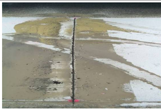
Image C. Spalling of joints due to tender mix or fibers or a combination of both.
