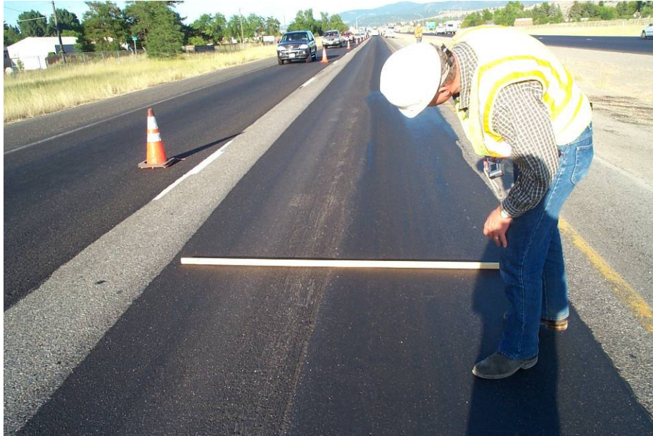
Image 3. Micro Surfacing placed as a rut fill prior to Macro-Surfacing within the two westbound lanes of I-90 (MP 293.15 to MP 293.55).
