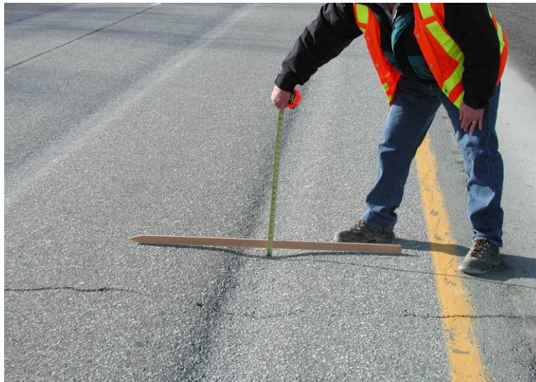
Figure 1. Studded tire wear in HMA pavement on I-90 near the Idaho border.
