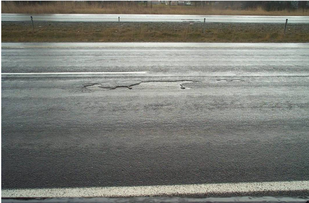
Figure 20. Pop out in the macro-surfacing. Photo taken in January 2005.
