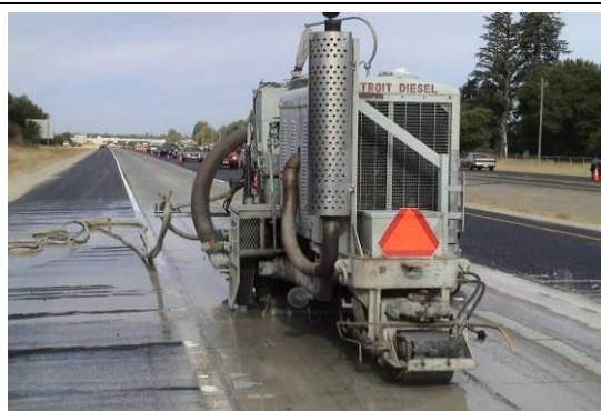
Image E. Diamond grinding to remove the ruts from the vehicle that entered the construction zone.
