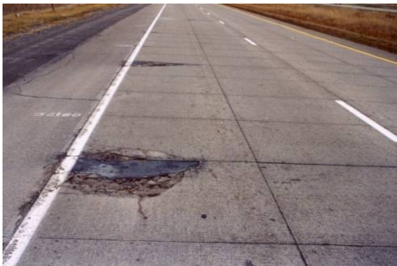
Figure 22. Cracking in MnROAD Test Cell 95, 3 inch whitetopping with a 5 ft by 6 ft joint spacing. Photo courtesy of Mn/DOT.
