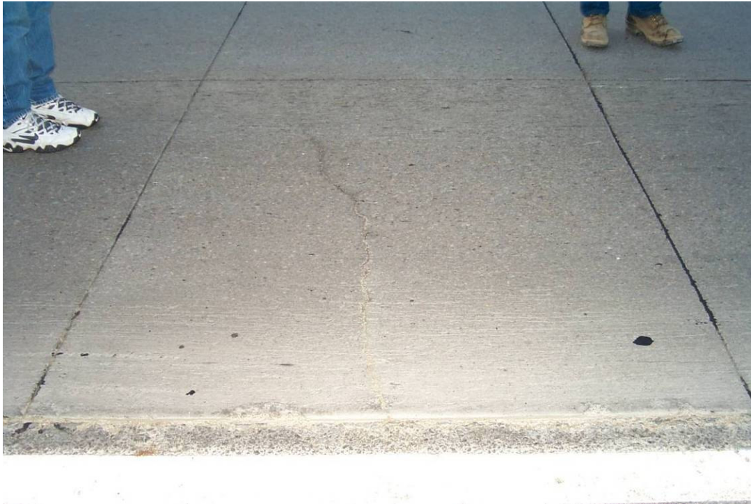
Figure 16. Mid-panel transverse crack in 5 inch test section.
