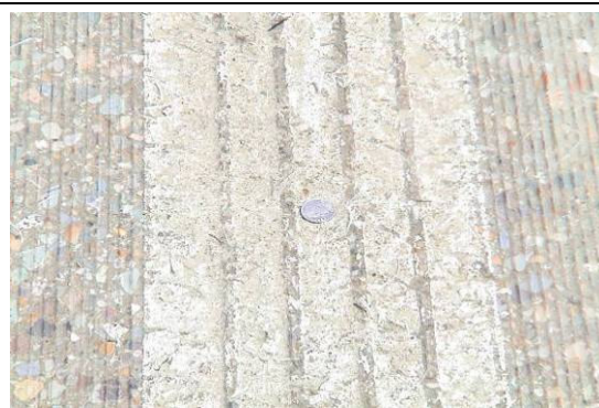
Image F. Ruts caused by vehicle that entered the construction zone during paving.
