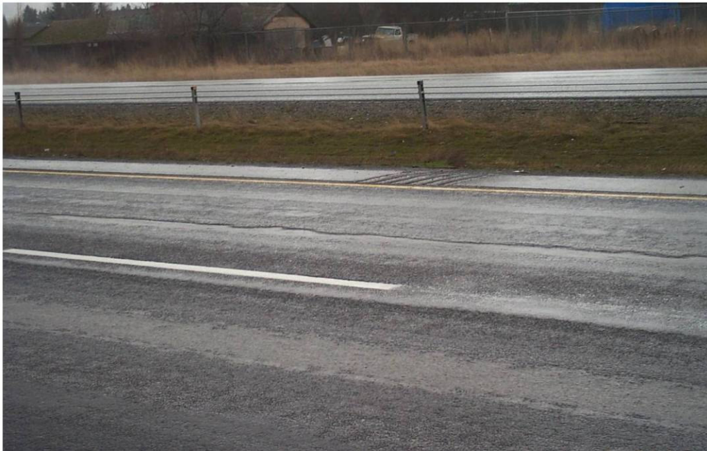
Figure 19. Delamination of the macro-surfacing. Photo taken in January 2005.
