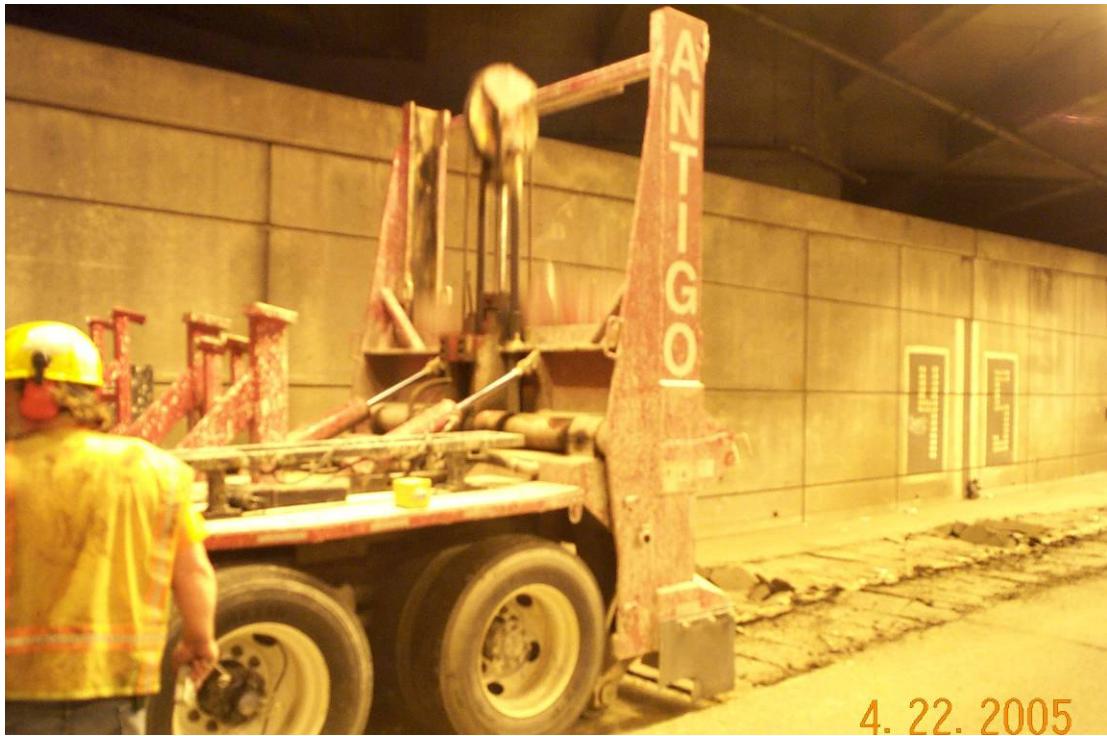
Figure 9 - Truck mounted drop hammer breaking PCC pavement under the Washington State trade and Convention Center (Photo courtesy of WSDOT).
