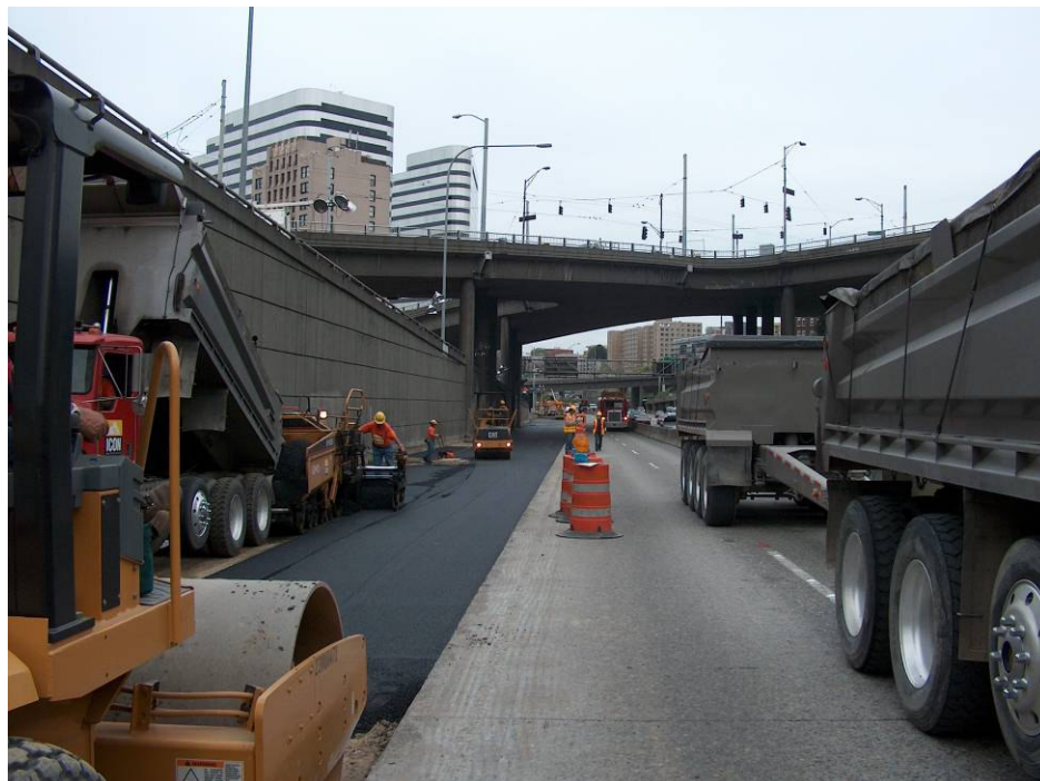
Figure 12 - Delivery, placement and compaction of HMA pavement with one access lane (Photo courtesy of WSDOT).
