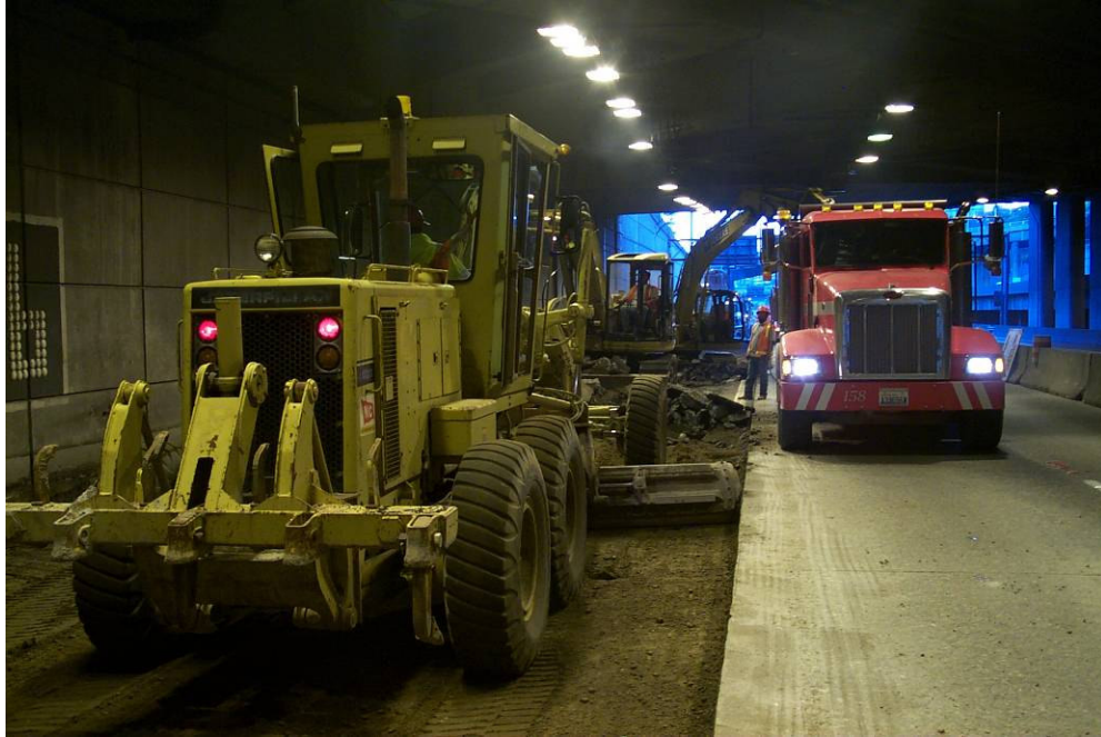
Figure 11- Removal of excess subgrade and subgrade preparation for HMA placement. Trucks were confined to one access lane immediately adjacent to paving lanes (Photo courtesy of WSDOT).
