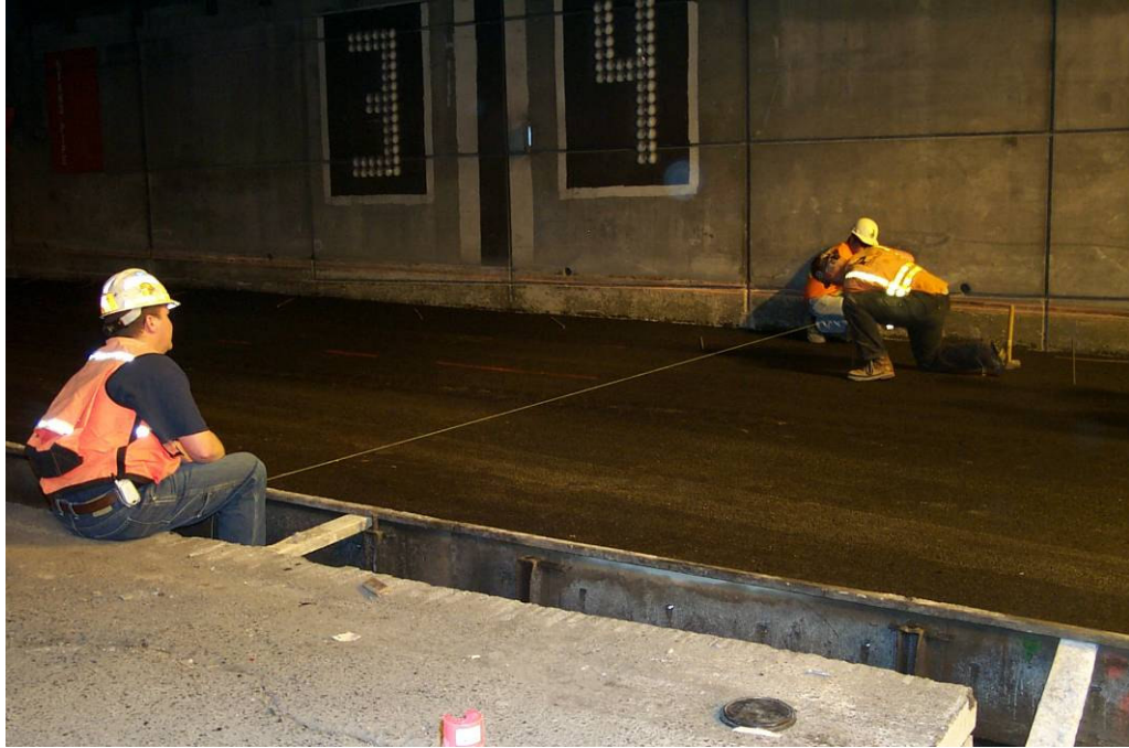
Figure 13 - Setting up forms and checking widths prior to PCC paving (Photo courtesy of WSDOT).
