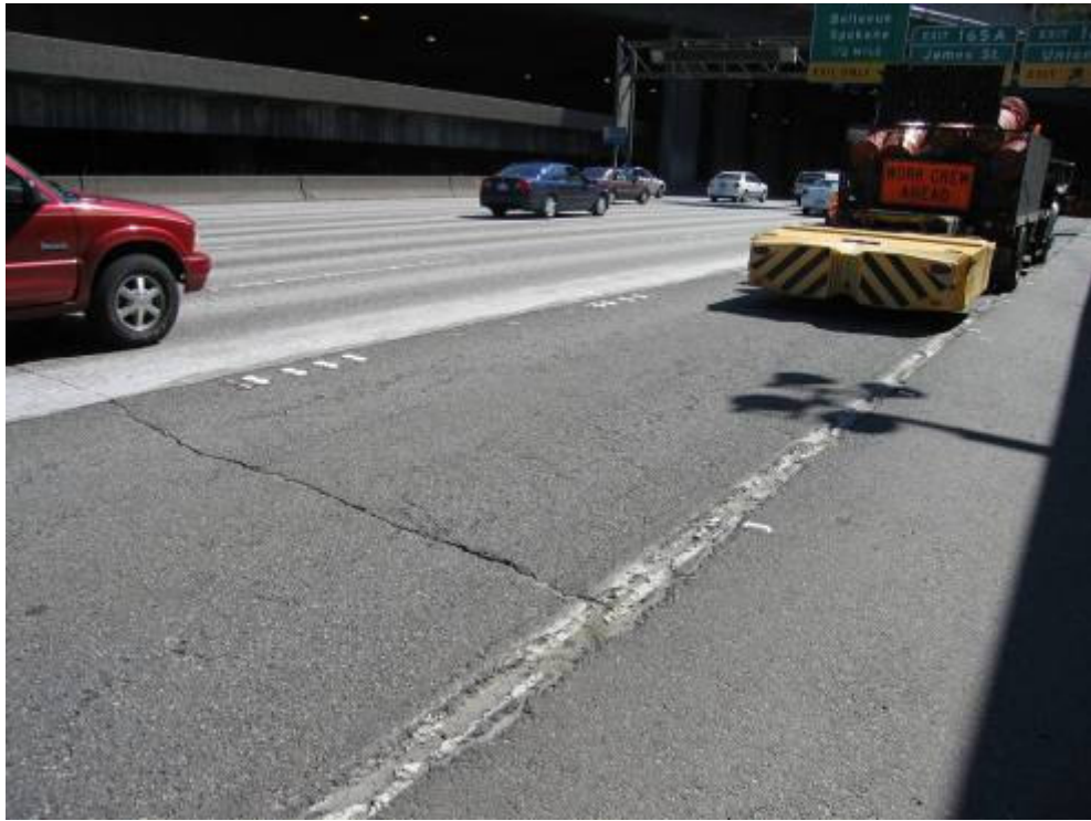
Figure 7 – Fatigue cracking and wear prior to project construction (Photo courtesy of WSDOT).
