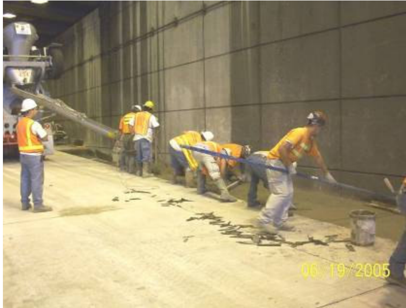
Figure 18 - Hand paving operations working against a structural wall (Photo courtesy of WSDOT).
