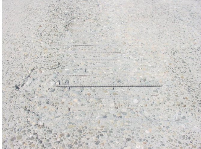
Figure 41 - Exposed bridge reinforcement steel Puyallup River Bridge. (Tharp, 2004)
