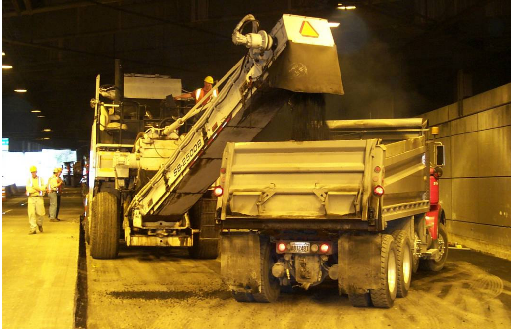
Figure 19 - HMA material transfer vehicle loading HMA truck in the construction pit (Photo courtesy of WSDOT).
