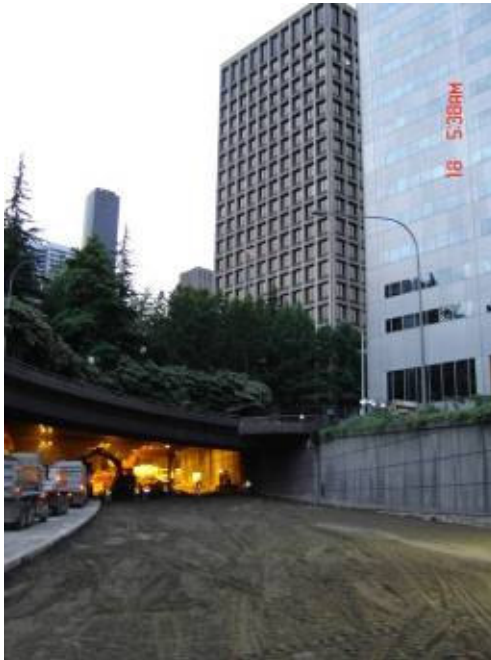
Figure 21 - Construction crews working under the convention center adjacent to commercial development (Photo courtesy of WSDOT).
