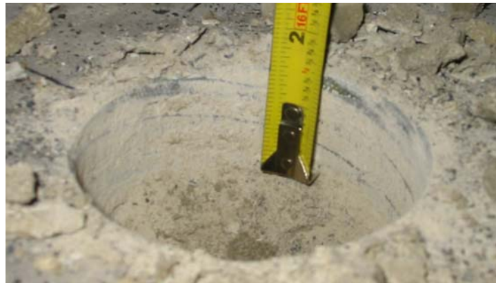
Figure 4.16: Grout damage: 08N08
