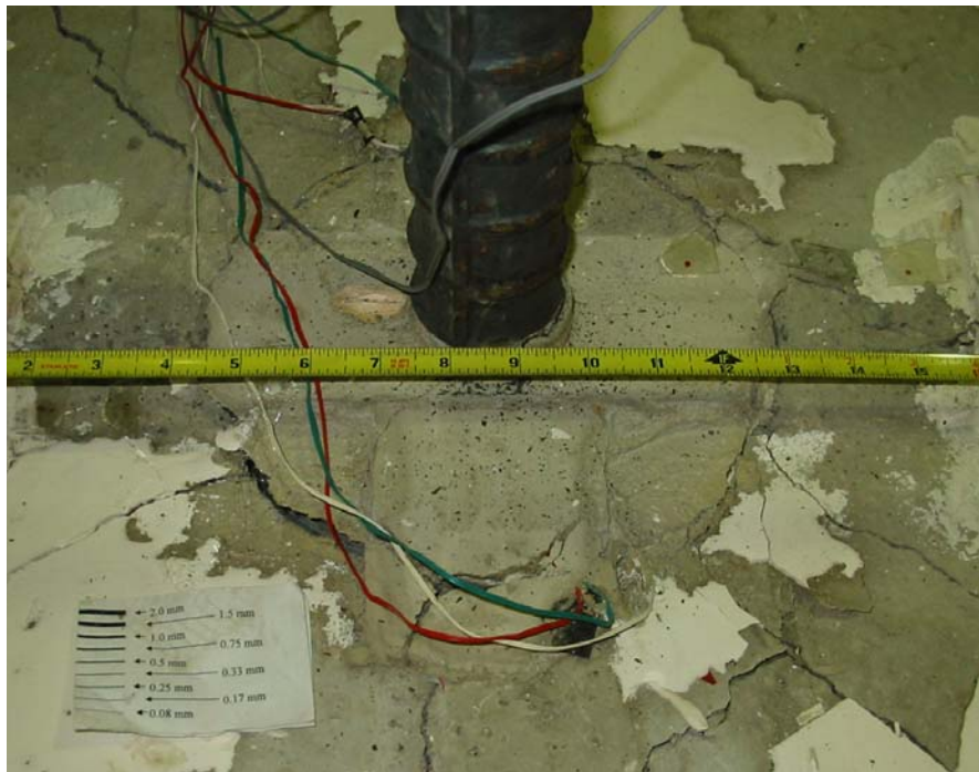
Figure 4.13: Concrete splitting: 18S04
