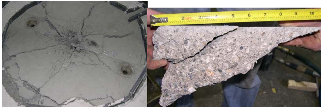
Figure 4.15: Concrete damage: 08C08
