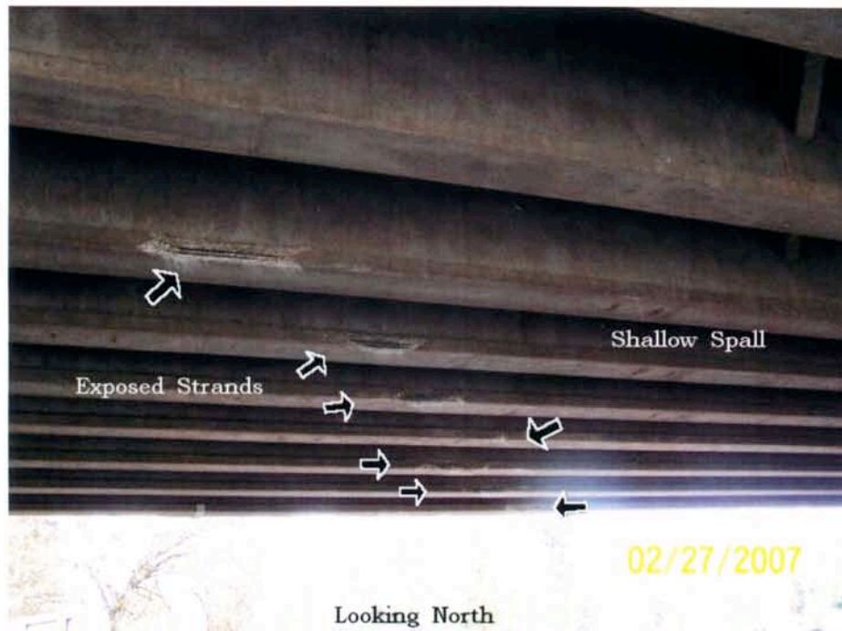
(c) Comparison with the observation from the real scenario – spallation of front faces at the bottom of girders
