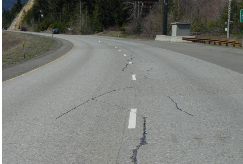
Figure 28 Longitudinal cracking caused by failed tape joint.
