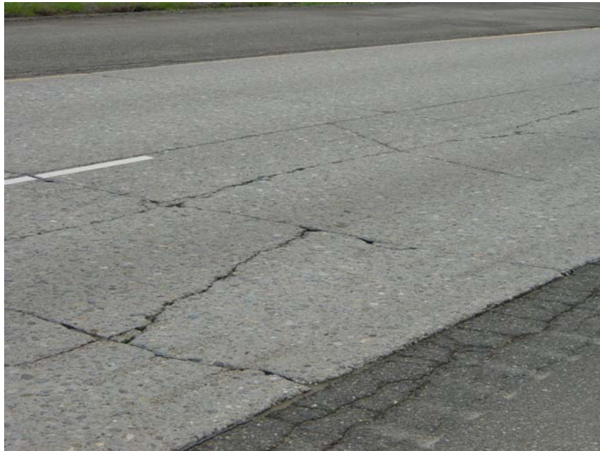
Figure 154 Test section – multi-cracked slab.
