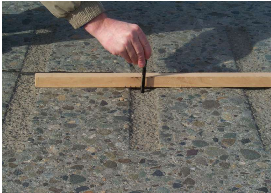
Figure 199 Studded tire wear of grout in dowel bar retrofit slot.
