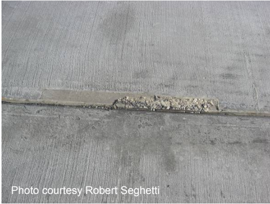
Figure 39 Spall to be repaired.
