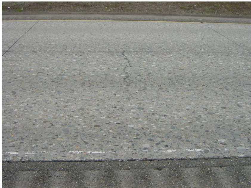
Figure 195 Transverse cracking after dowel bar retrofit.
