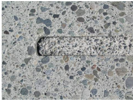
(c) Dowel bar slot debonding.
