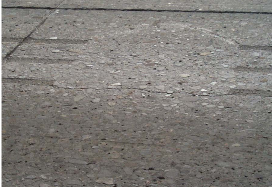
Figure 197 Longitudinal cracking after dowel bar retrofit.
