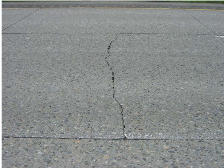
Figure 152 Test section – transverse cracking.
