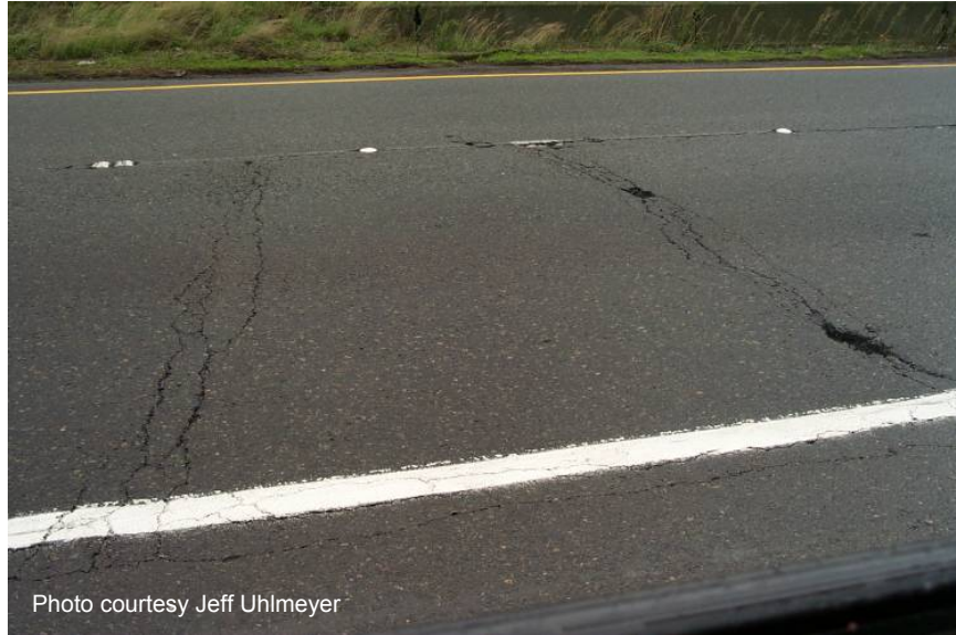
Figure 106 Reflection cracking (I-5 Centralia vicinity).
