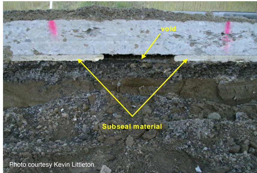
Figure 33 Uneven support of subseal operation.
