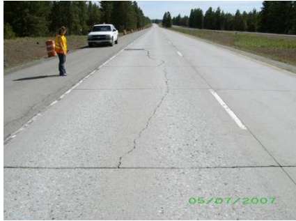
(a) Longitudinal cracking.
