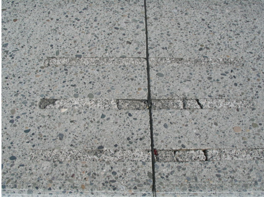
Figure 200 Patching material cracking.
