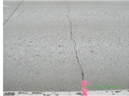
(b) Transverse cracking.
