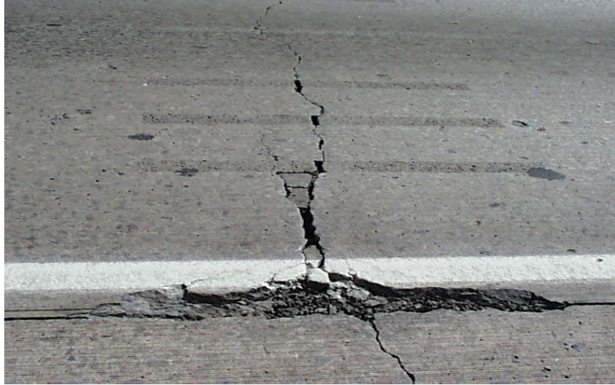
Figure 136 Spalling of dowel bar retrofitted transverse crack.
