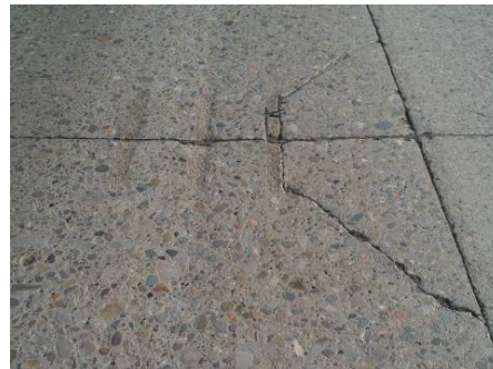
d. 45-degree cracking
