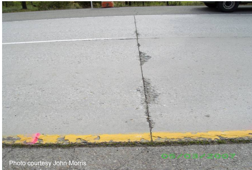
Figure 18 Spalling at a transverse joint.
