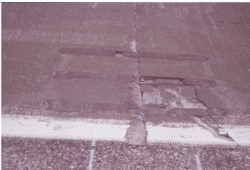
Figure 134 Cracking between dowel bar slots.
