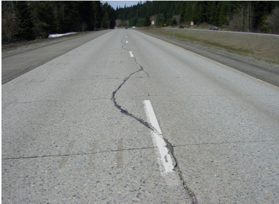
Figure 179 Failed longitudinal tape resulting in longitudinal cracking.
