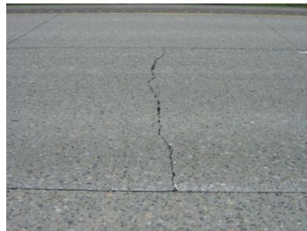
b. Transverse cracking
