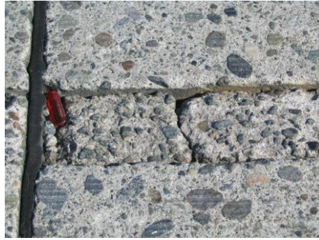
(b) Dowel bar slot cracking.
