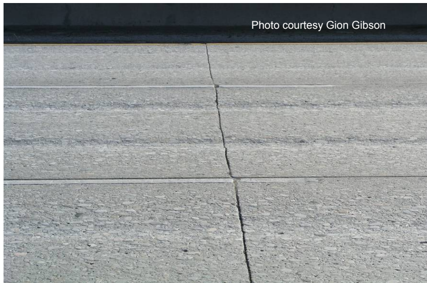
Figure 15 Severe studded tire wear (I-90 Spokane).
