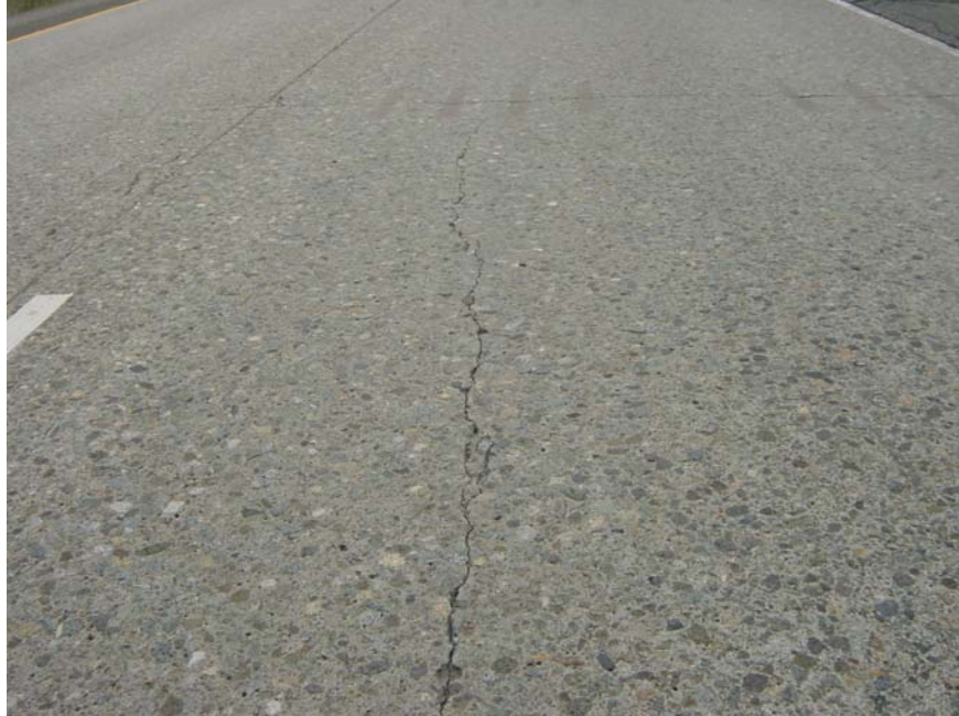
Figure 153 Test section – longitudinal cracking.
