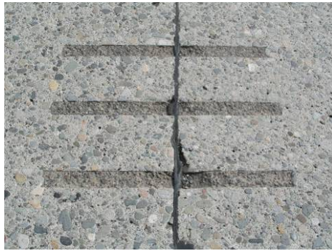
(a) Dowel bar slot spalling.
