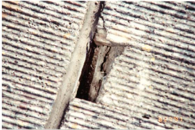
Figure 119 Typical distress caused at core board failure (Dunn et al., 1998).
