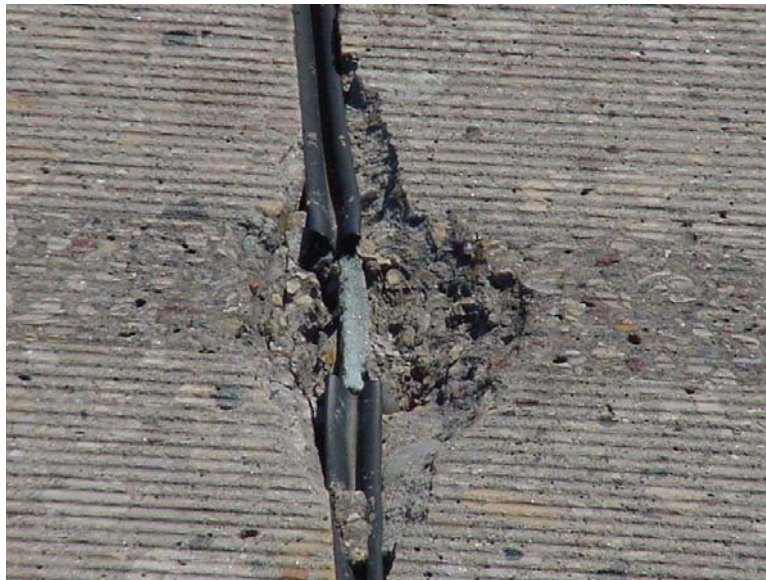
Figure 122 Mortar deterioration and spalling (Wilson et al., 2002).
