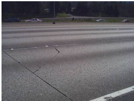
c. Corner cracking
