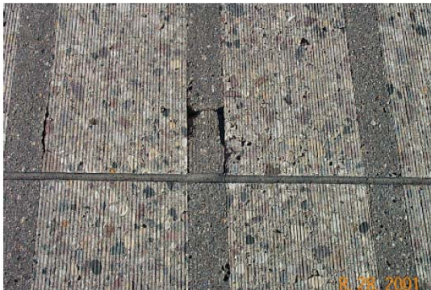
Figure 121 Typical distress in Patchroc 10-60 (Dunn et al., 1998).
