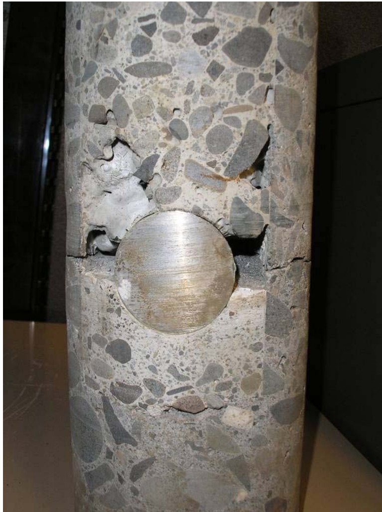
Figure 213 Poor consolidation of patching material around dowel bar.
