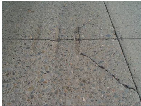
(e) 45-degree cracking.
