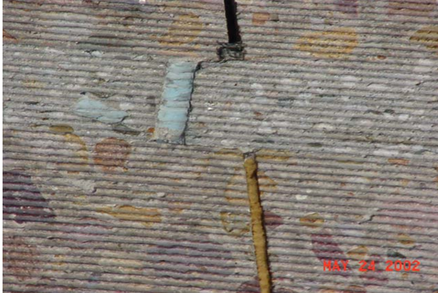
Figure 128 Misaligned foam core board State Route 8 (Glauz et al., 2002b).
