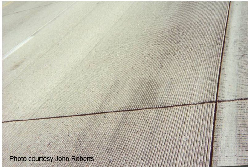
Figure 68 Diamond grooved surface.
