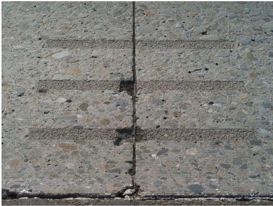
Figure 204 Spalling of patching material.
