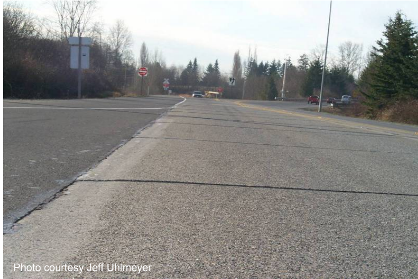
Figure 19 Transverse joint faulting.
