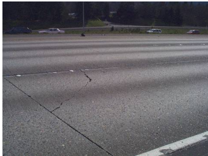
(c) Corner cracking.
