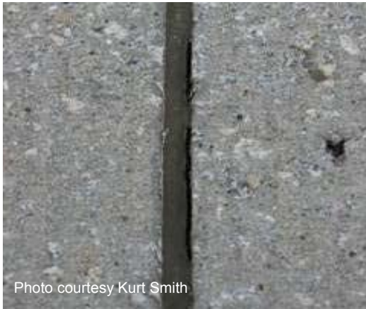
(a) Adhesive failure.
