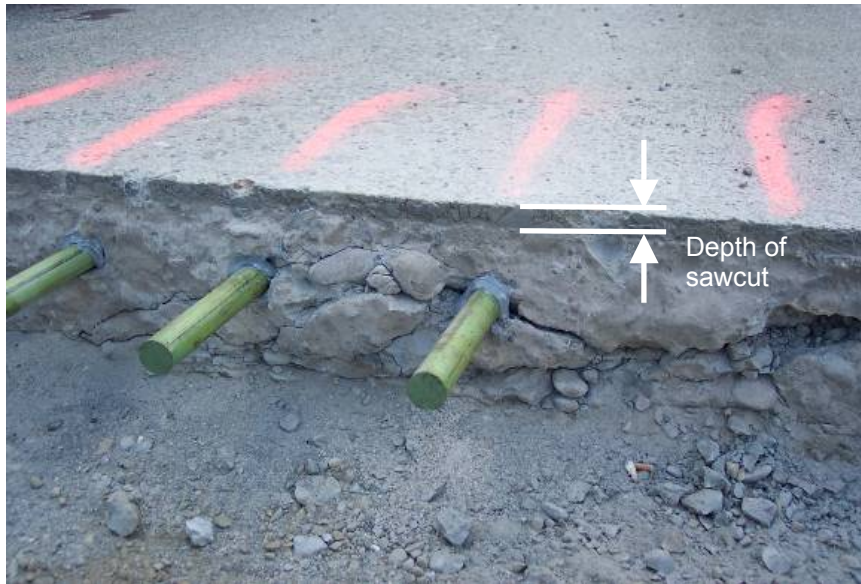
Figure 236 Panel not sawcut full-depth.
