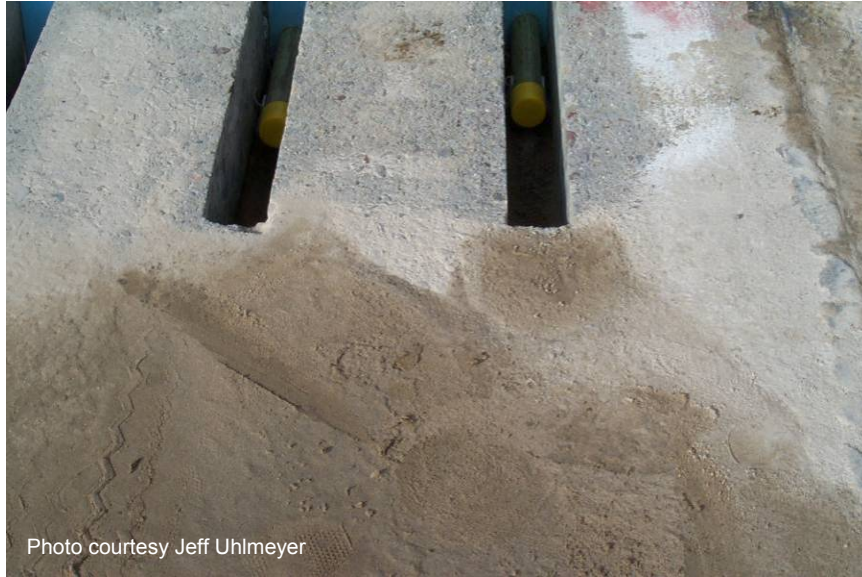
Figure 124 Debris left adjacent to dowel bar slots.
