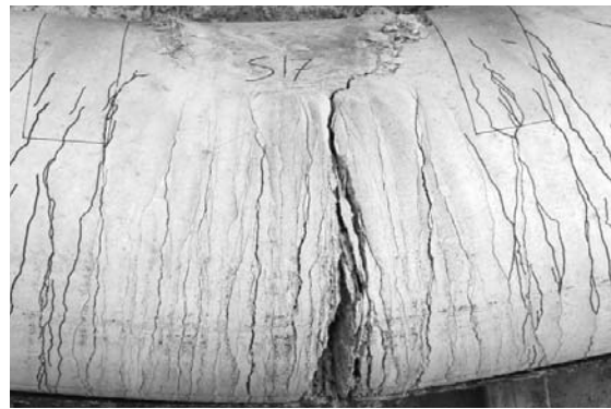
b) Flexural Cracking of Concrete Fill
