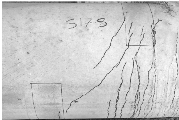
c) Limited Diagonal Shear Cracking of Concrete Fill
