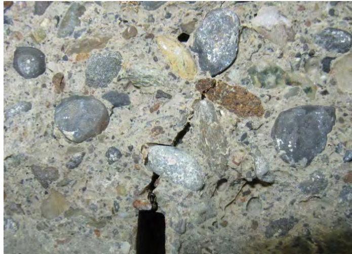
(a) Crack propagating path during fracture test
