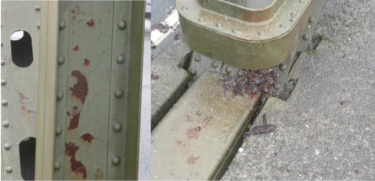
Figure 5. Sol Duc #5 Bridge with rough paint surface and problem area where girder meets the deck
