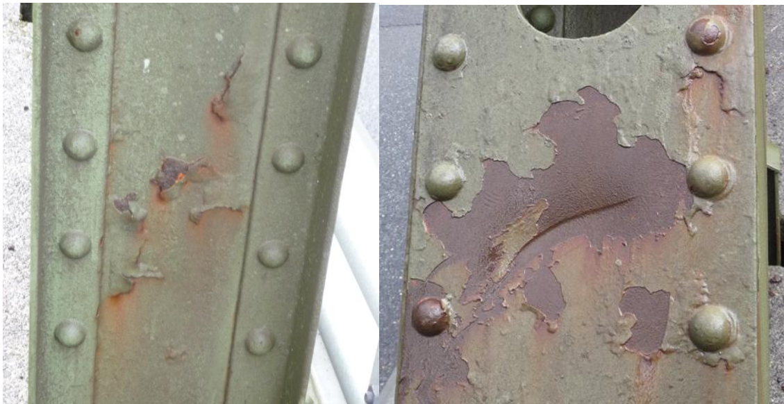
Figure 4. Sol Duc #4 Bridge with rough paint surface and motorist damage
