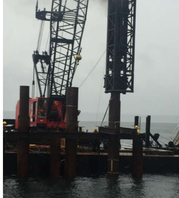
Figure 3b. The three piles in the template, taken on 8 December. The control pile is on the left, the double wall pile is in the middle, and the mandrel pile is on the right.
