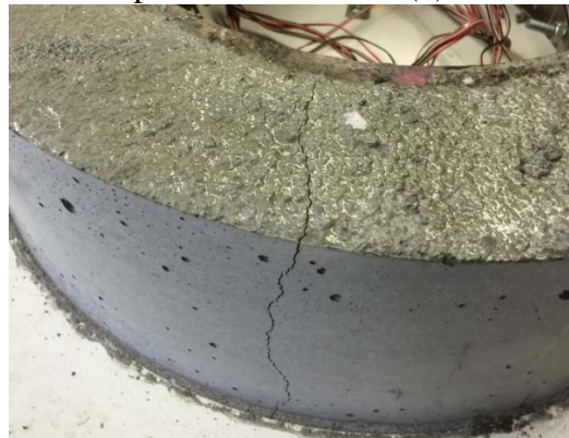
(e) Typical shrinkage cracking
