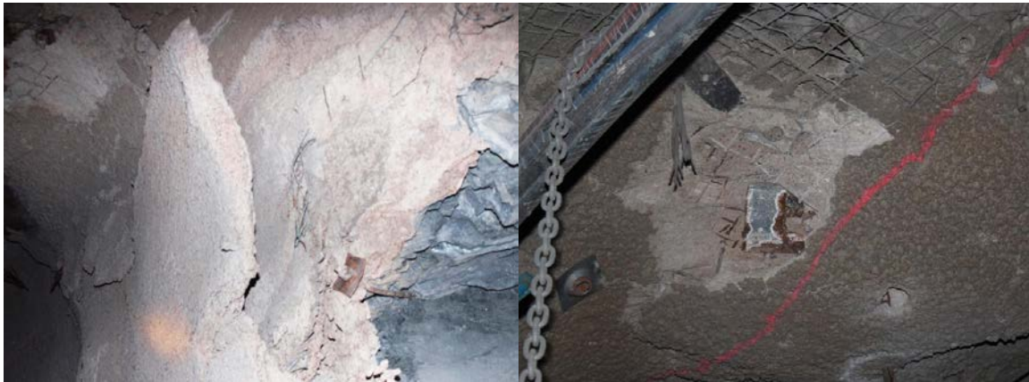
Figure 1.3 Debonding issues of shotcrete (Drover and Villaesusa, 2015)
