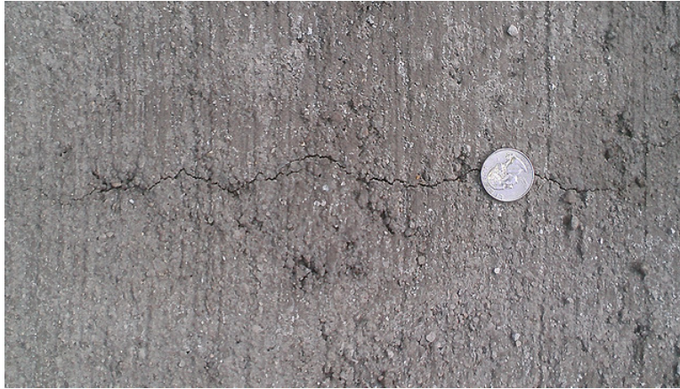
Figure 1.2 Observed early-age shrinkage cracking in shotcrete structures
