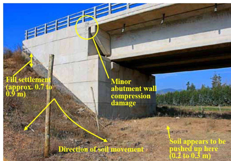
Figure 3.1: Settlement and lateral spreading deformation of northeast approach embankment to Mataquito River Bridge (FHWA, 2011).
