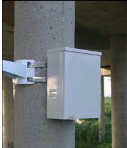
Figure 5.1: Metal case mounted on a light pole for MUST-II installation
