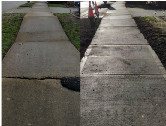
$100 million funding level. (Left): Sidewalk before pedestrian improvements. (Right): Sidewalk after pedestrian improvements.
