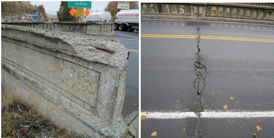
Examples of deteriorated bridges that could become unusable with continued underfunding.
