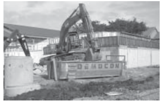
The demolition contractor removes concrete from the old Merrill Hall floor. All concrete will be reused in the project.
