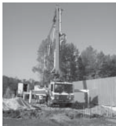
A concrete truck pumps concrete into the new foundation at Merrill Hall.
