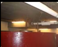
6" Air gap (at King Street Center)
