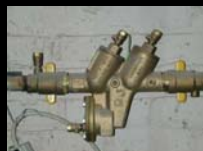
Reduced pressure principle backflow assembly
