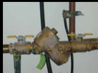
Double check valve backflow assembly
