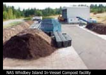
NAS Whidbey Island In-Vessel Compost facility
