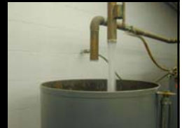
An air gap between rainwater cistern and potable back-up
