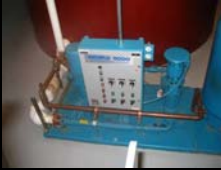
Commercial pumping system
