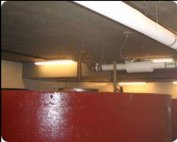
6" Air gap (at King Street Center)
