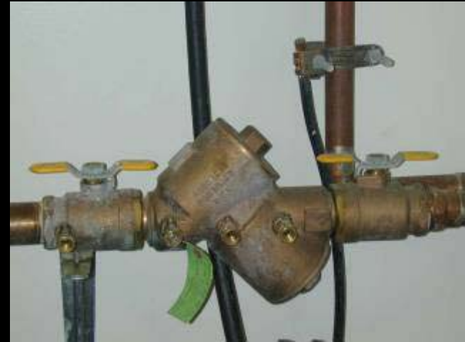
Double check valve backflow assembly
