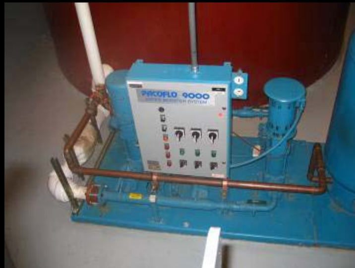
Commercial pumping system
