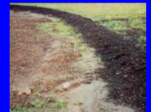
Berms instead of silt fence
