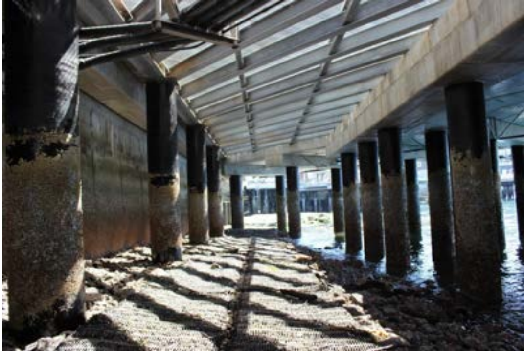
Figure 4. Underneath the rebuilt Pier 62 at low tide, showing light through the grating.
