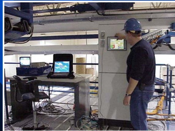
Integrated Control System
