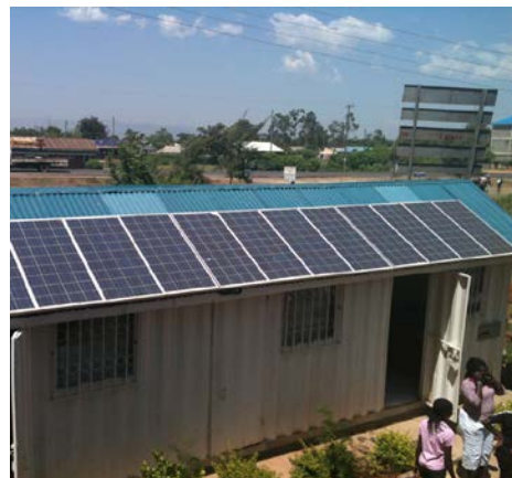
CFAR supported the installation of solar panels to power computer and laboratory equipment in a small research building at the Ahero sub-district hospital in rural Western Kenya, where power outages are common.
